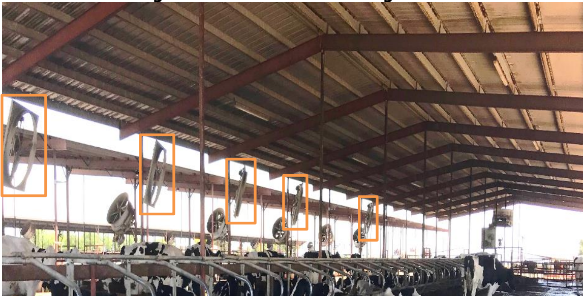
Figure 5: Fans Used for Cooling in Pen
