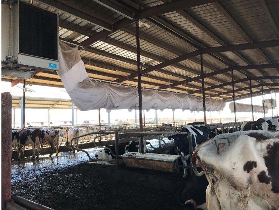
Figure 6: Targeted Convection Cooling System
