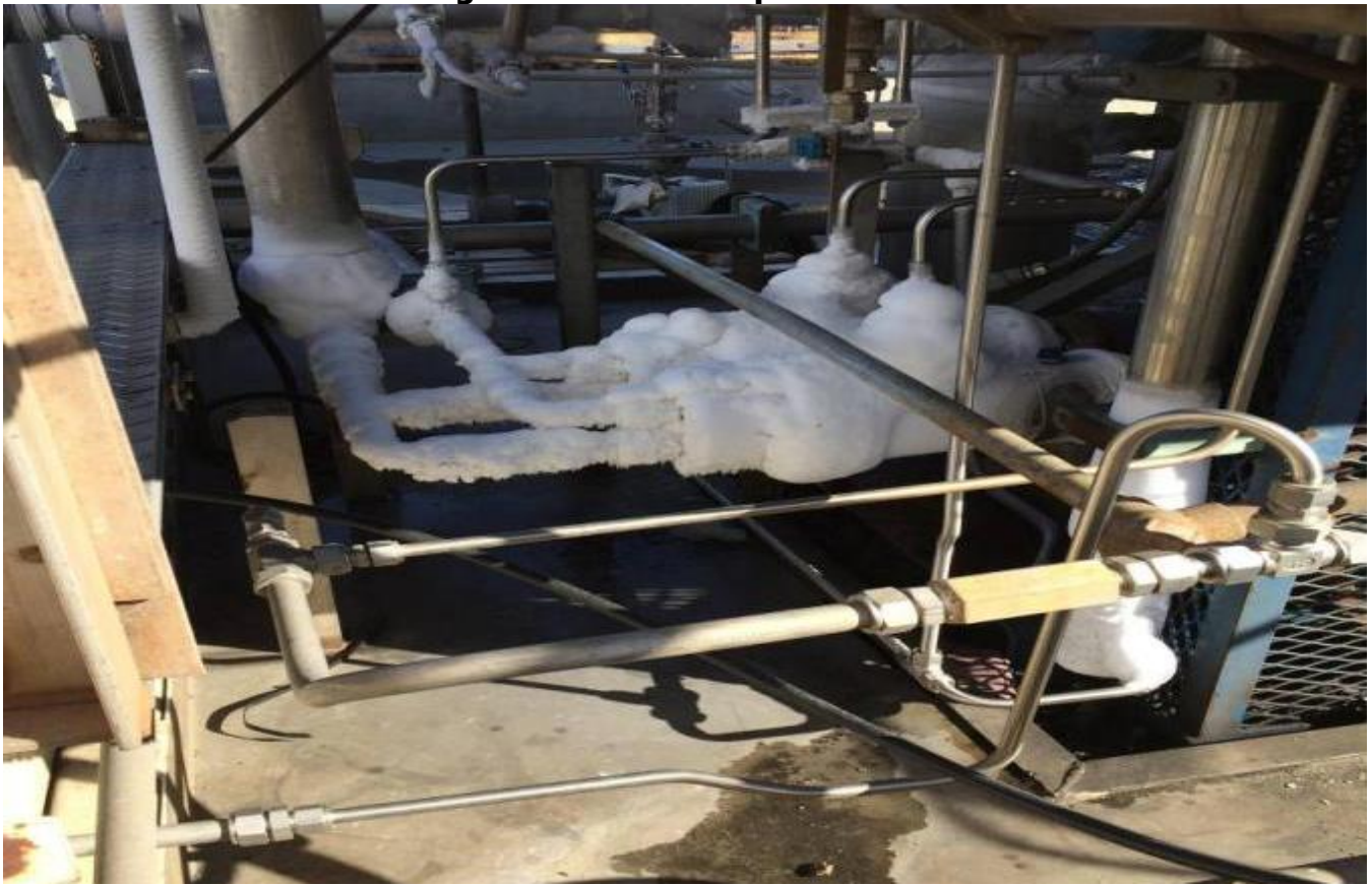
Figure 7: LCNG Pump Cold Ends
