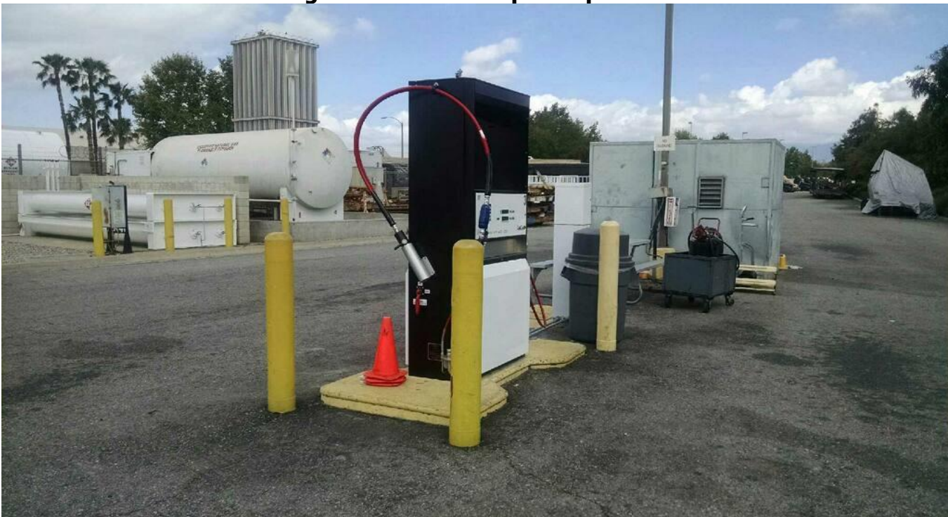
Figure 8: CNG 3600 psi Dispenser
