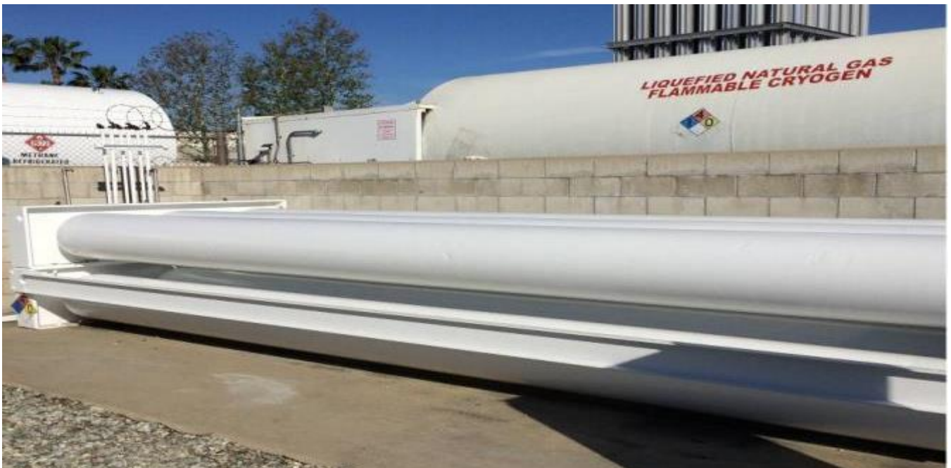
Figure 6: CNG Vessels Corrosion Control and Paint
