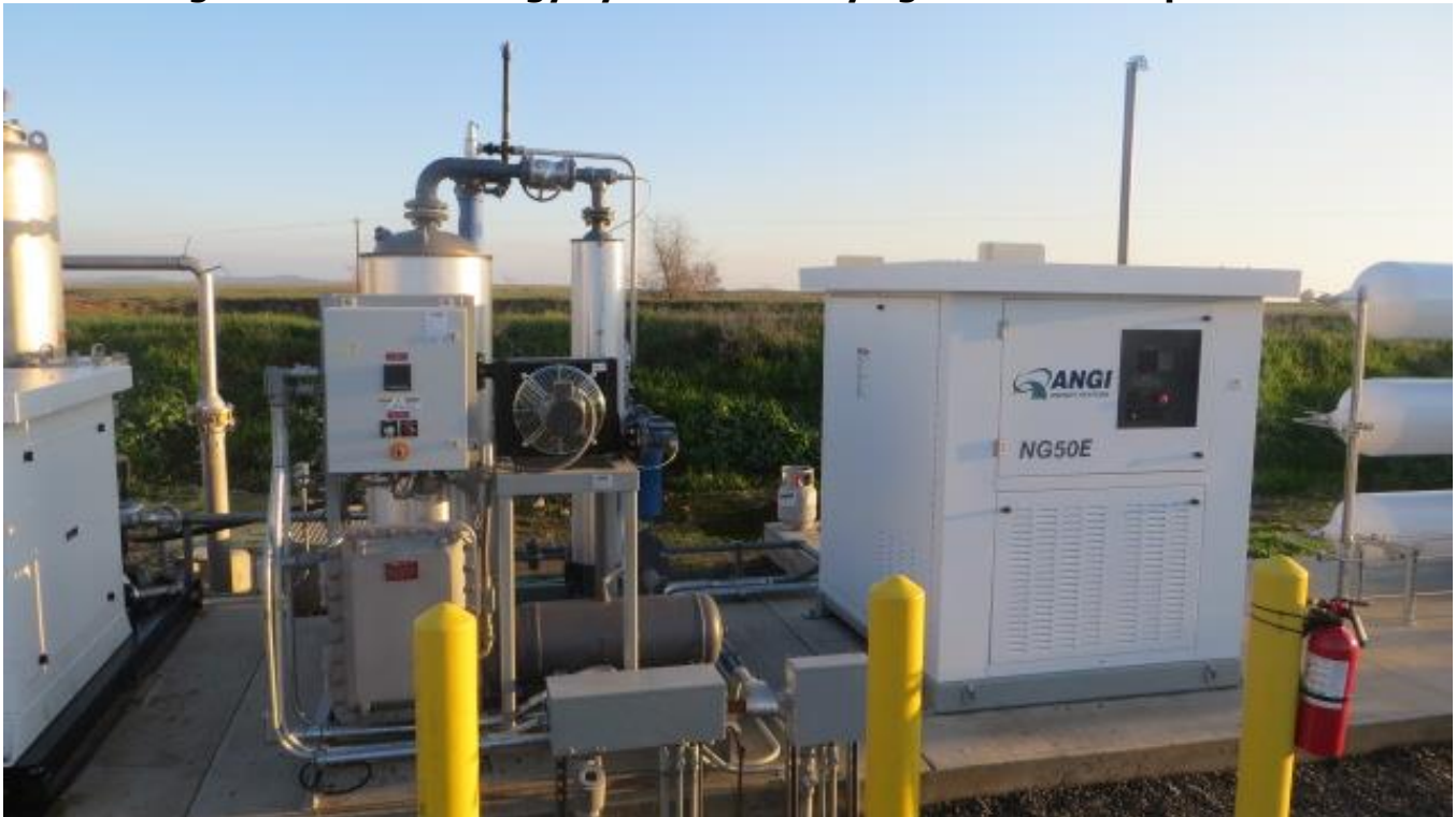
Figure 11: ANGI Energy Systems LLC Drying Skid and Compressor
