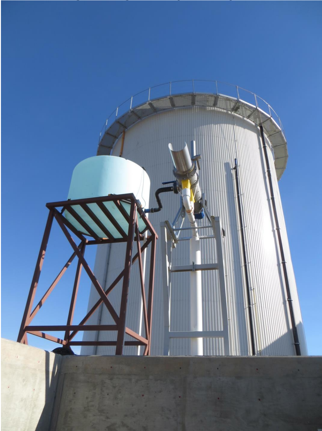
Figure 5: Digestate Separation System
