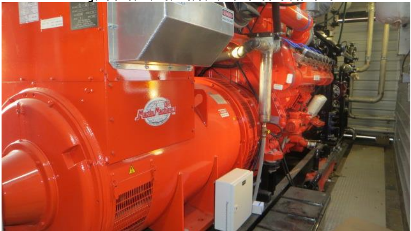
Figure 8: Combined Heat and Power Generator Unit
