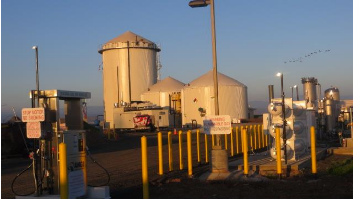
Figure 13: CNG Dispenser and Anaerobic Digestion Equipment
