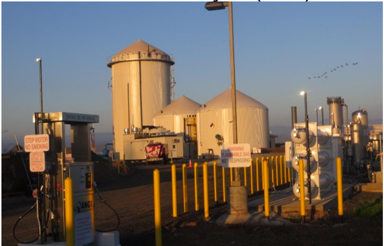
Figure ES-1: North State Rendering's Completed Anaerobic Digestion Project with Renewable Natural Gas Fueling Station (lower left)
