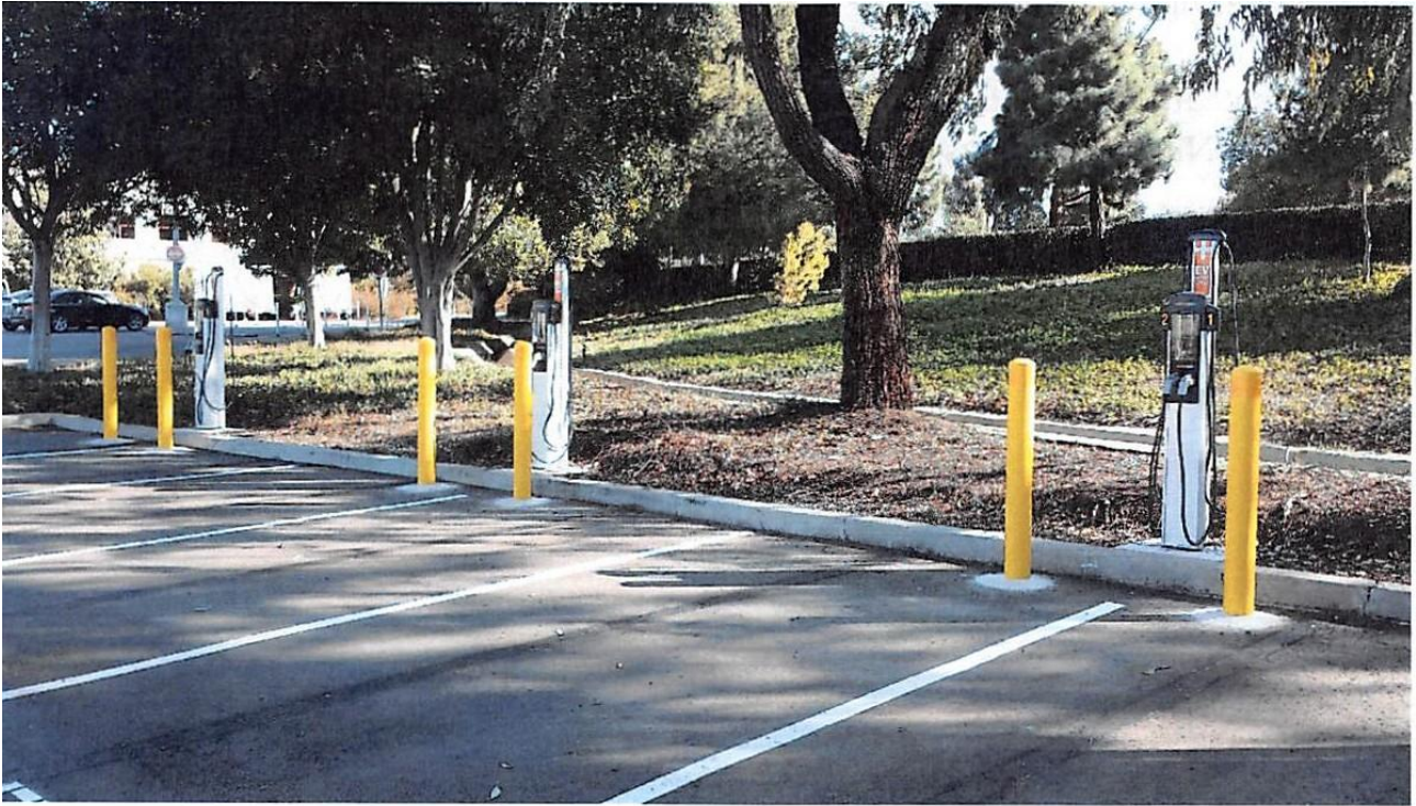
Figure 3: MSTB Site Post EVSE Installation
