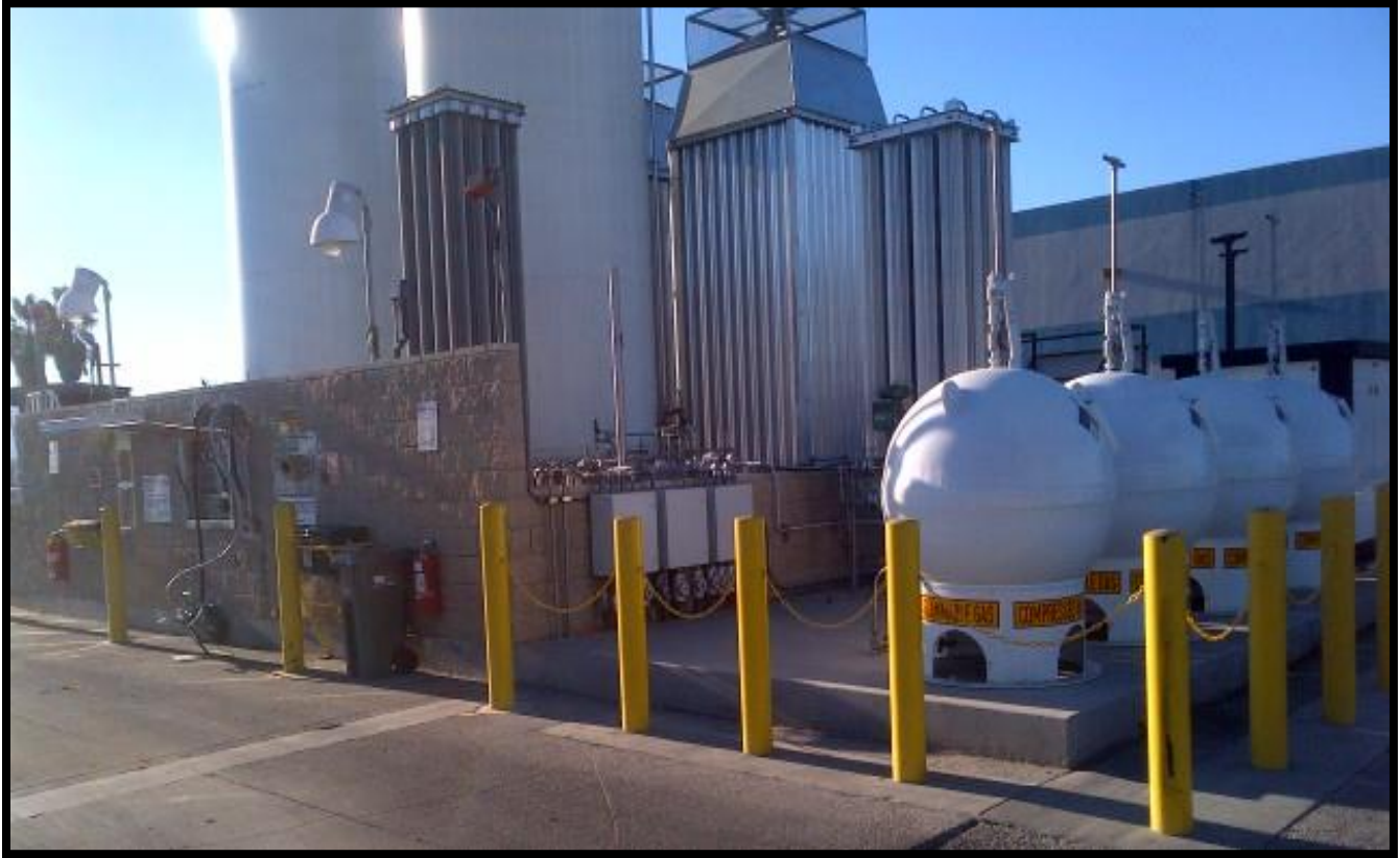
Figure 3: Side View of Station Showing CNG Storage Spheres and Vaporizers
