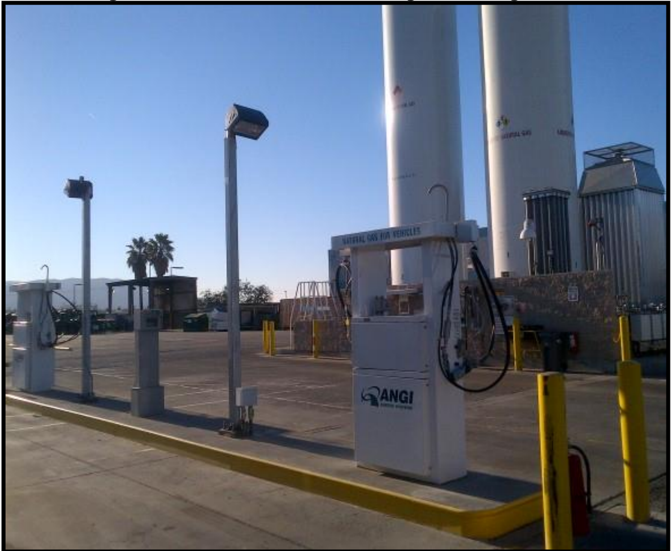
Figure 2: Front View of Station Showing CNG Fueling Island
