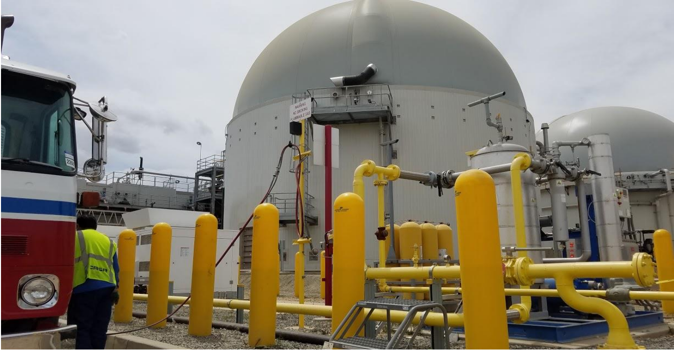
Figure 6: CNG Fuel Charging Station
