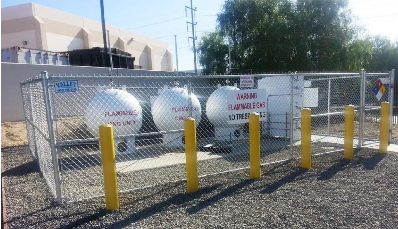
Figure 3: New Storage Vessels and Priority Valve Panel
