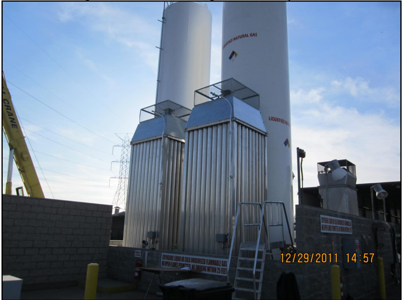
Figure 2: Side View of Storage Tanks and Vaporizers
