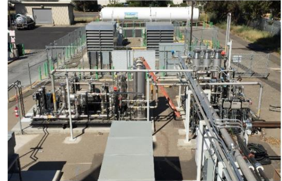
Final biogas processing system (4.17.15)
