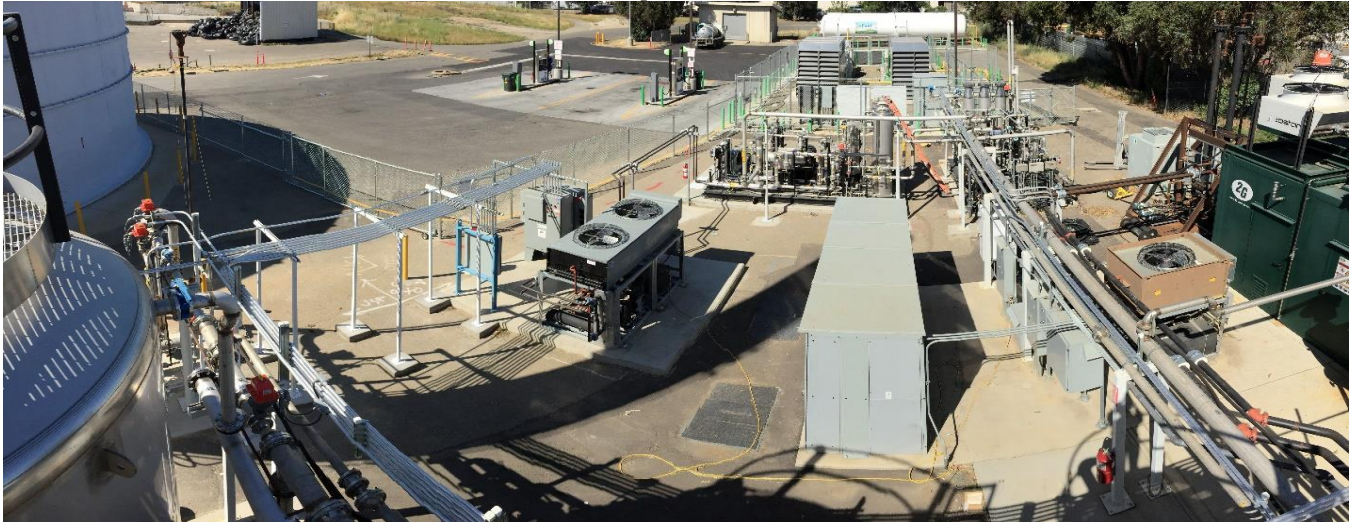
Figure 10: Overview of Fully Installed Biogas Collection, Cleaning, and Conversion System
