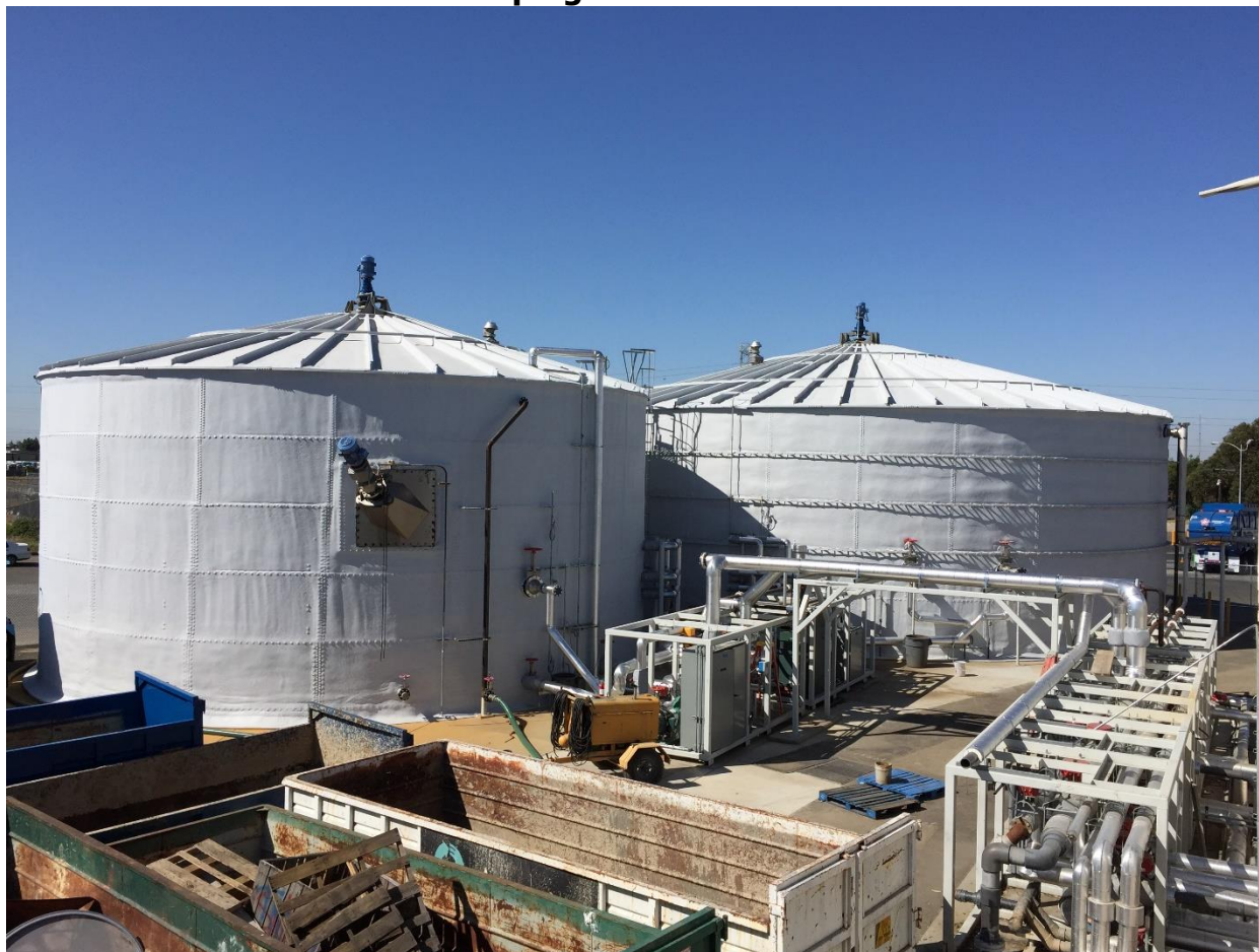
Figure 8: Fully Installed Tanks and Skids with Insulation and Completed Field Piping Connections
