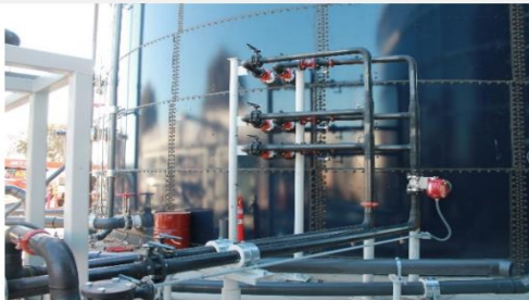
Hot water piping (9.30.15)
