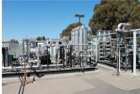
Second biogas processing system (9.15.14)
