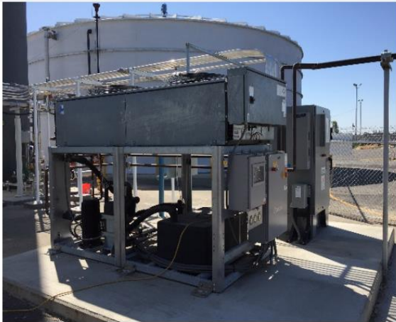
New biogas chiller (4.17.15)
