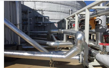
Final hot water piping (4.17.15)
