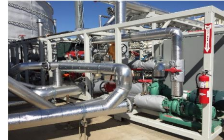
Final skid piping (4.17.15)
