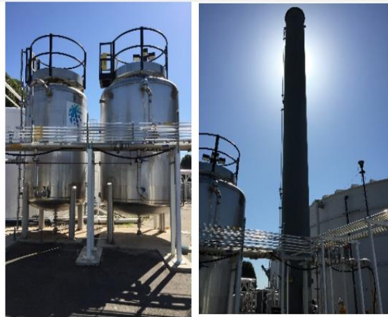
New H 2 S scrubbing system – left – and flare – right (4.17.15)
