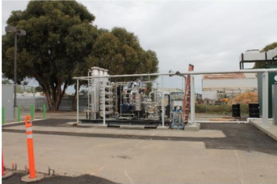
Original biogas processing system (2013)
