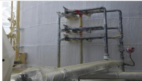
Hot water piping (3.2.15)
