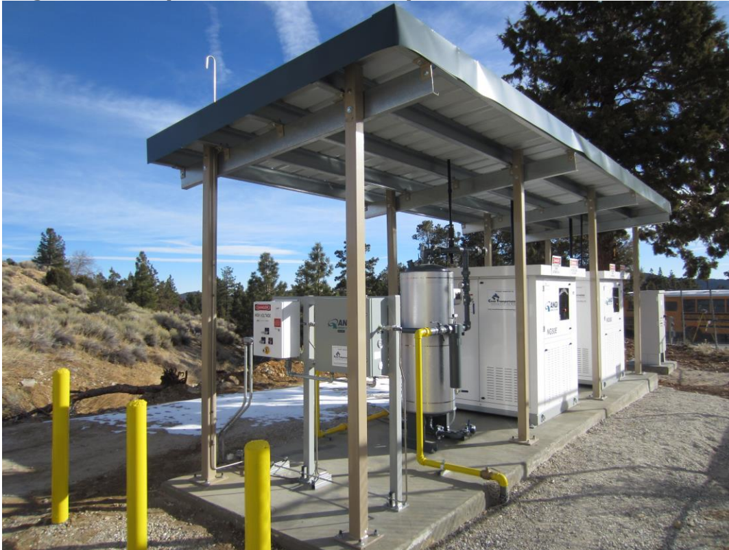
Figure 4: Completed CNG Station, Operational October 21, 2013
