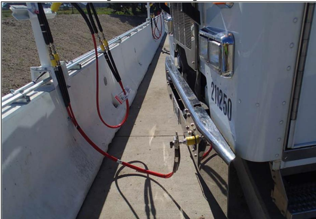
Figure 3: CNG Filling Stall
