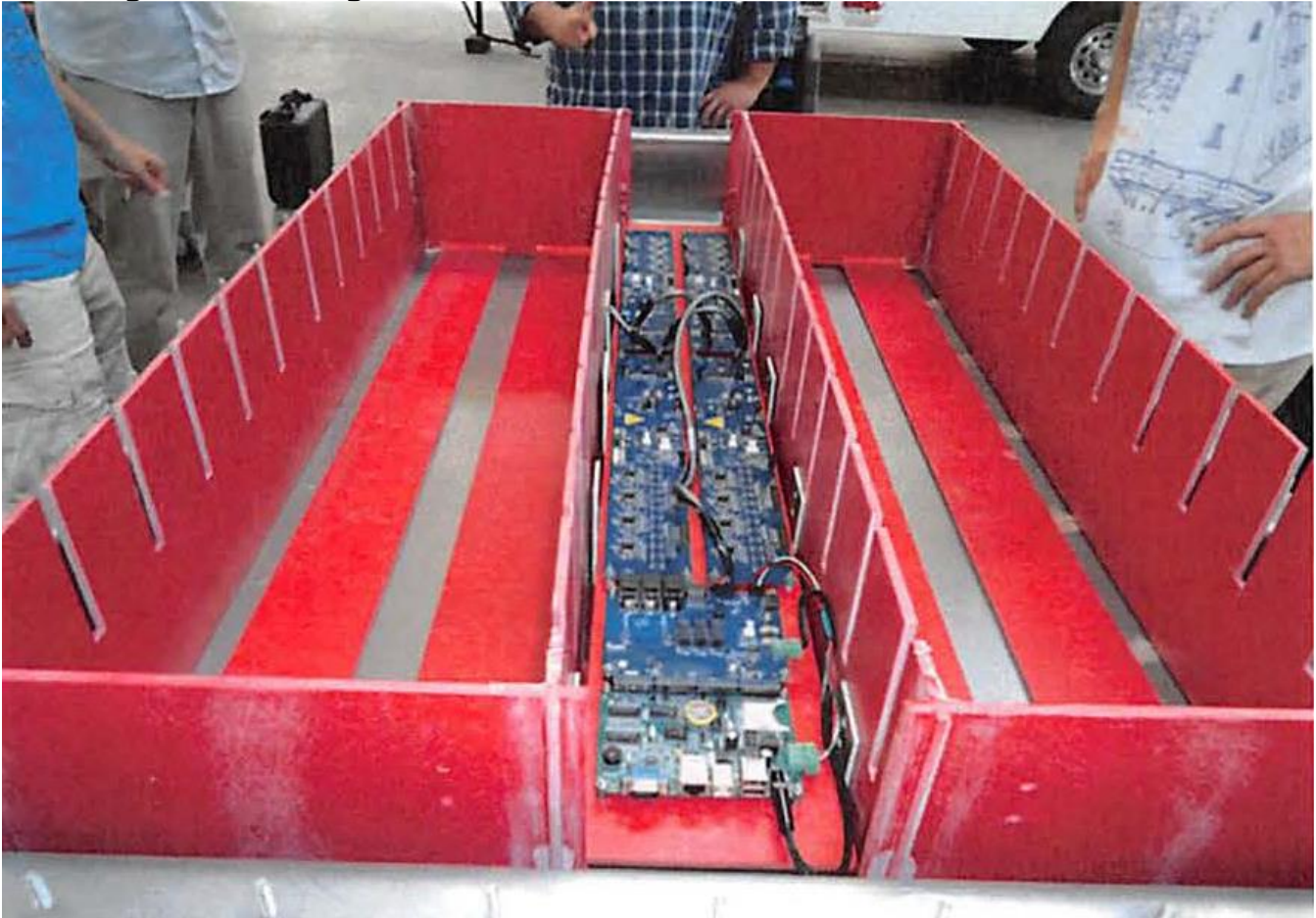
Figure 22: Fiberglass Base Plate with BMS Electronics Mounted in Place
