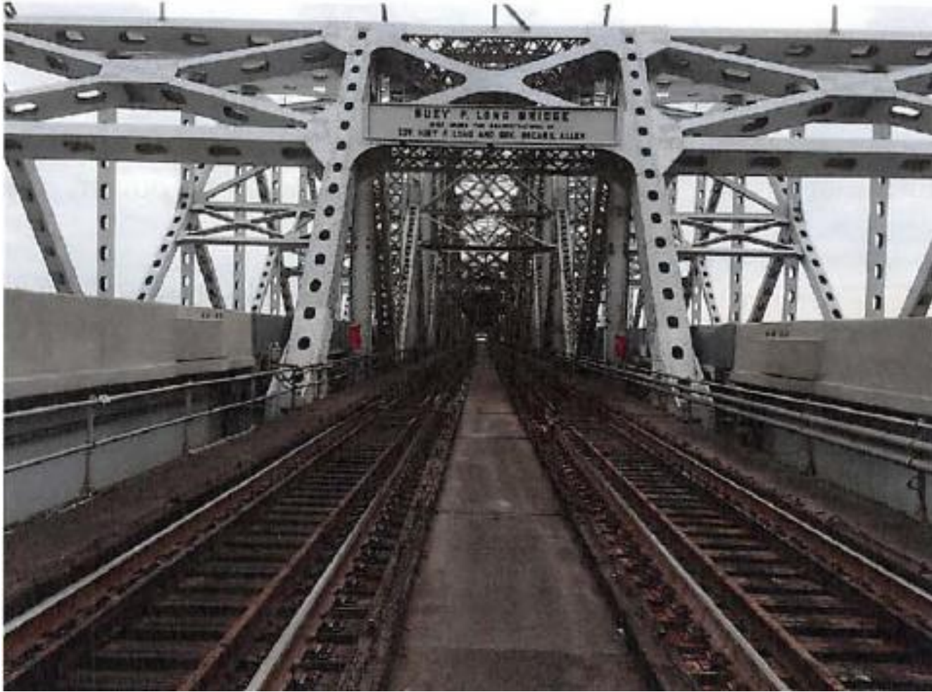
Figure 32: View of Huey P. Long Bridge Test Site in New Orleans, Louisiana.
