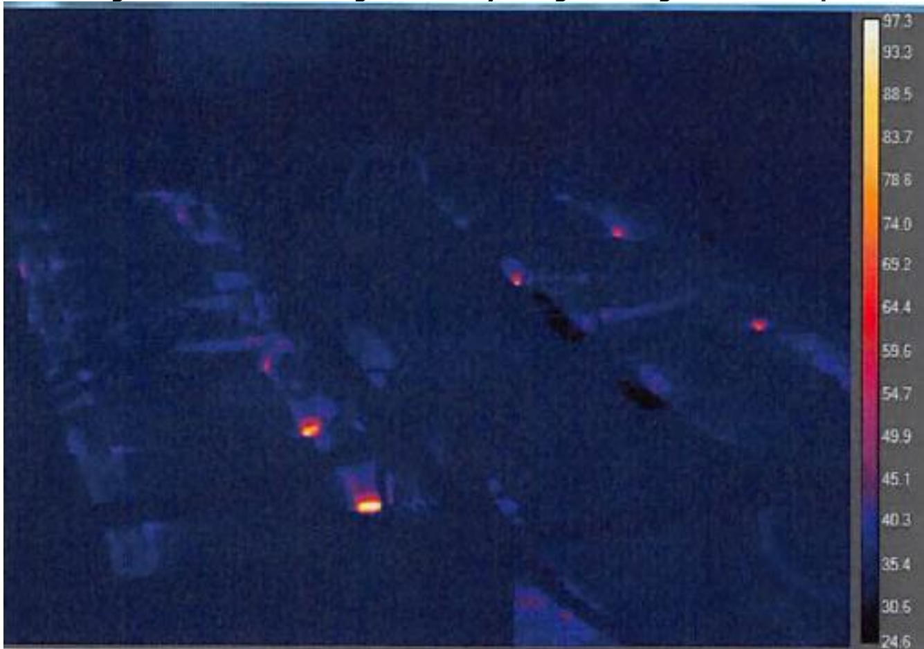
Figure 28: Thermal Image of Battery Being Discharged at 180 Amps
