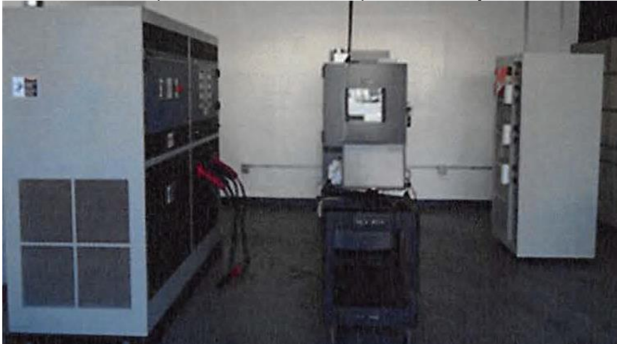
Figure 6: BMS Lab Equipment Installation Complete (From Left to Right: AV 900 HV, 1007C Thermal Chamber, NHR-9200 LV)
