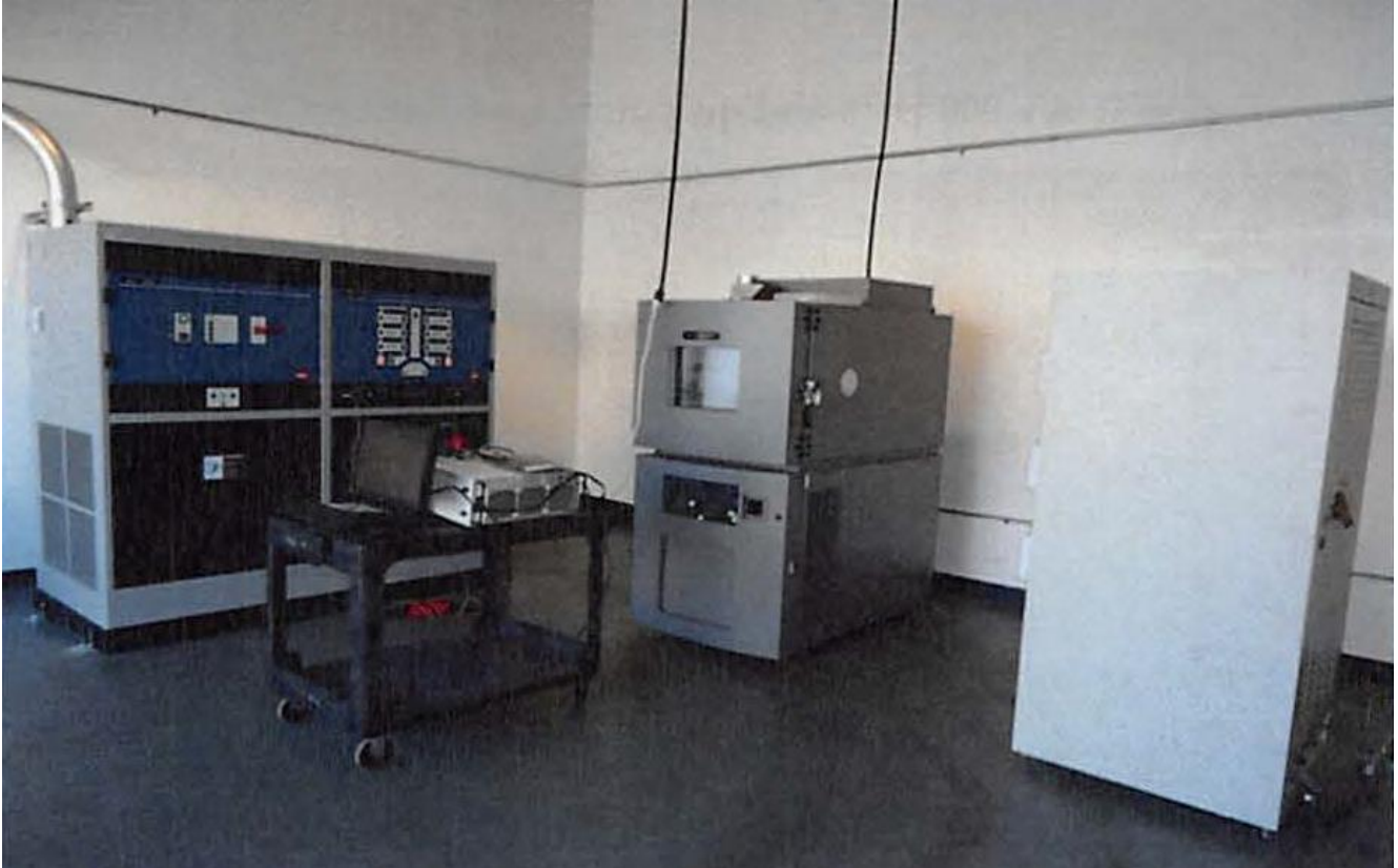
Figure 7: Another View of BMS Lab Equipment Installation Completed (Note PC and DAQ on cart)
