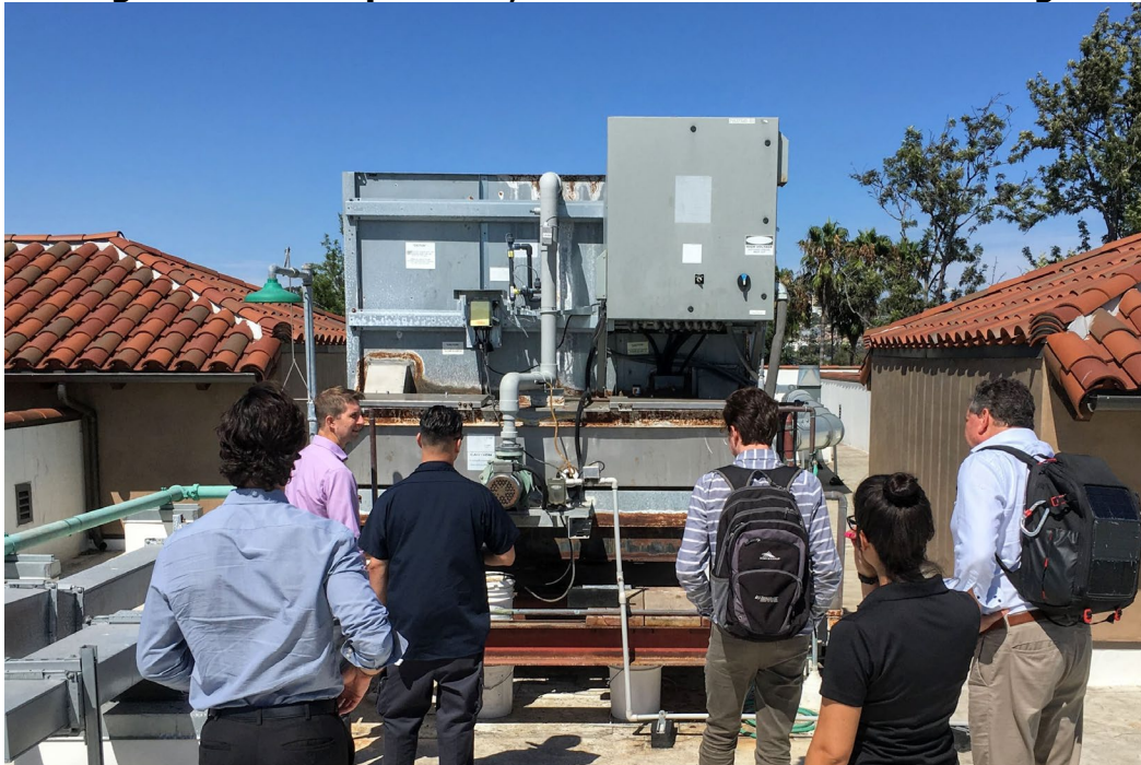
Figure 4: Rooftop Chiller, Hilton Garden Inn in San Diego
