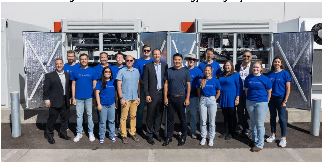
Caption: Smartville MOAB™ Energy Storage System, powered by repurposed EV battery packs and charged by a UC San Diego solar energy array
