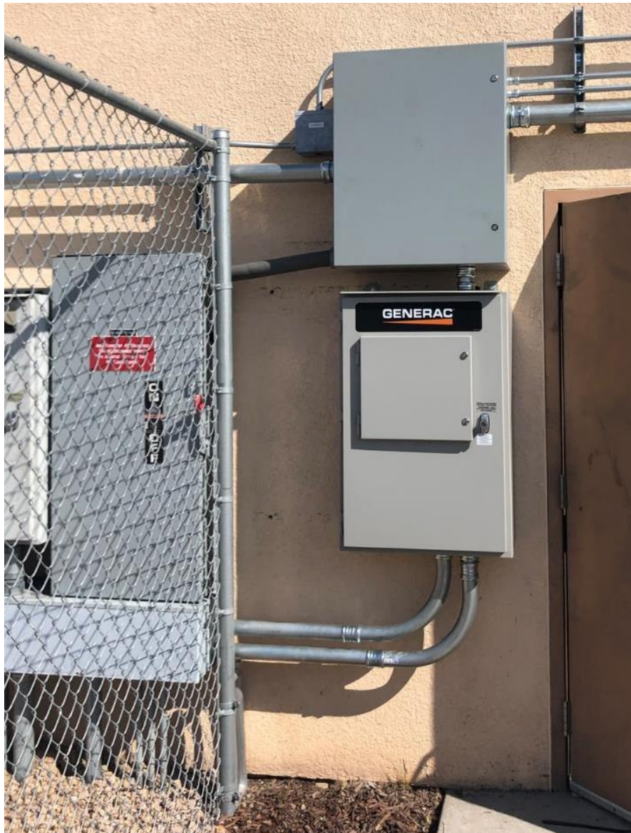
Figure 33: Replacement Grid Islanding Disconnect and New Automatic Transfer Switch
