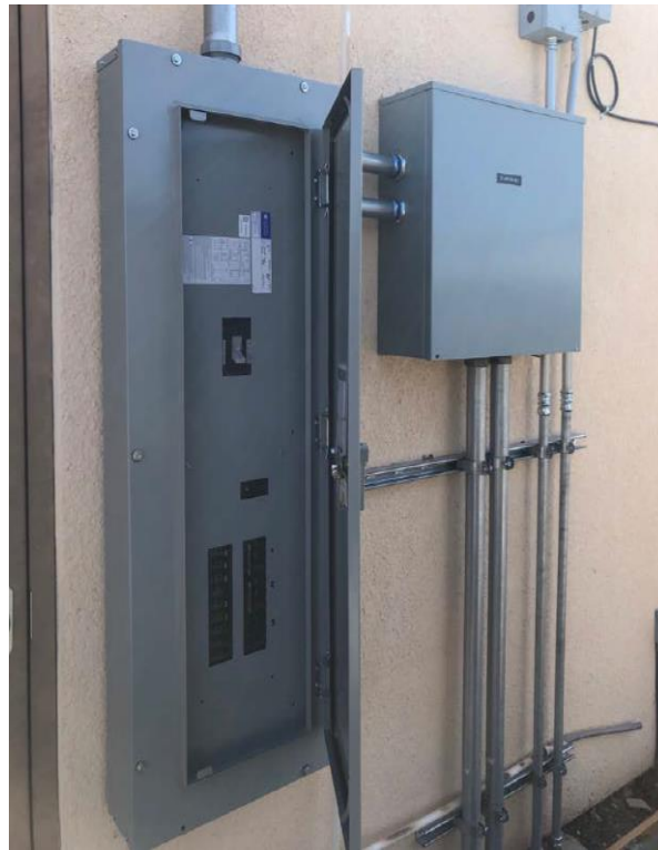
Figure 31: New AC Distribution Panel
