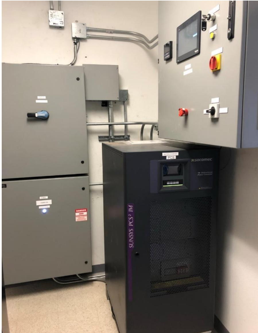
Figure 34: Battery Inverter and Controller Box
