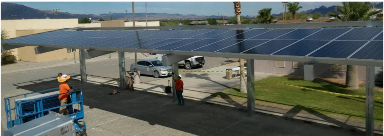
Figure 7: Solar Photovoltaic Carport Structure
