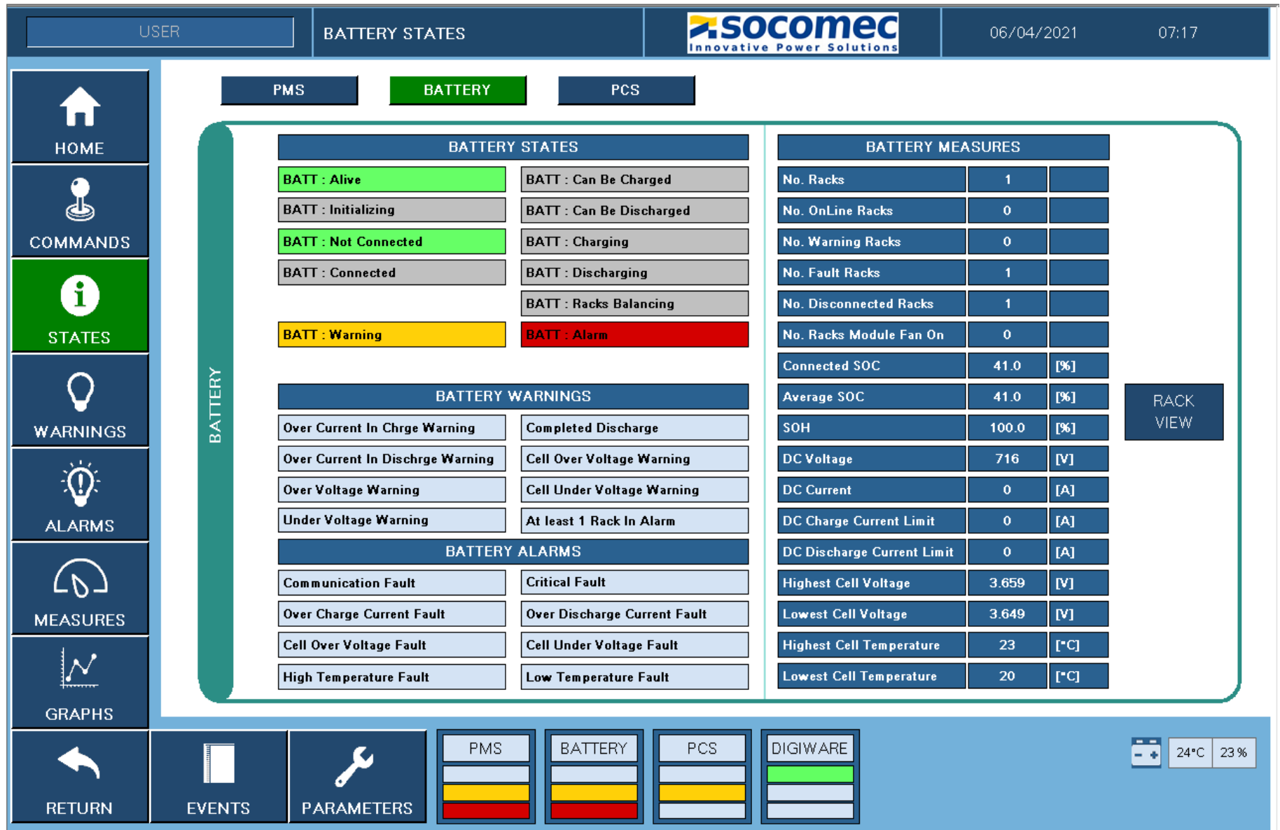
Figure 40: Socomec Battery Energy Storage System Controller Display
