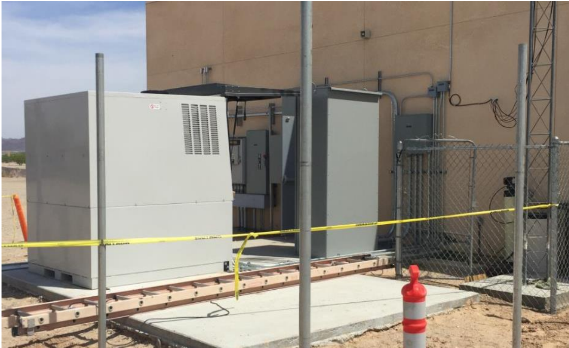
Figure 13: Battery Unit and Inverter Installed at Project Site
