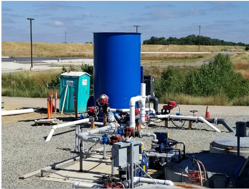
Biofiltration Skid with Completed Piping Connections.
