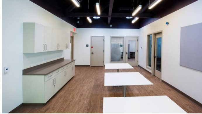
Figure 14: Interior Breakroom with Installed Tubular Daylighting Devices
