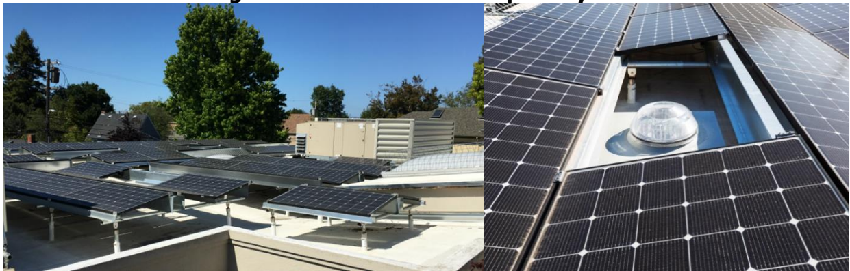
Figure 13: Installed Rooftop PV System
