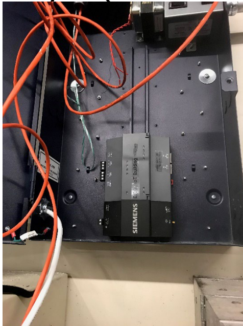
Figure 43: Global Controller for Heating, Ventilation, and Air Conditioning Control System (Siemens TNM 8000)
