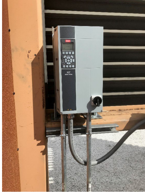
Figure 44: Variable Frequency Driver for Heating, Ventilation, and Air Conditioning Control System
