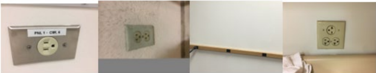
Figure 3: Outlets in Engineering and Computer Science Building
