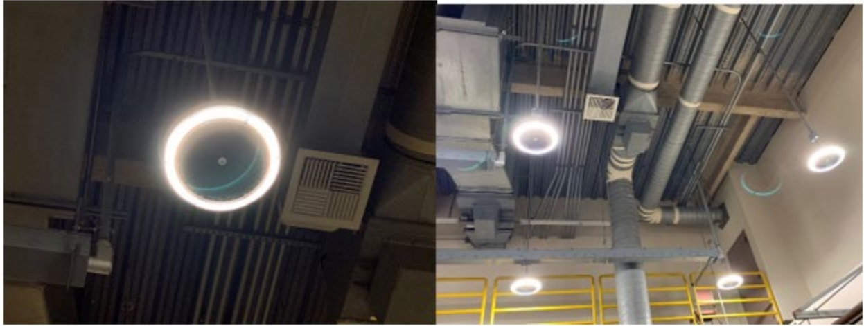
Figure 29: ILP UFO LED Installed in Engineering and Computer Science 111 (Chemical Lab Room)
