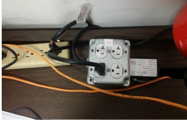
Figure 38: Enlighted Plug Load Controller Installed at Engineering and Computer Science 411
