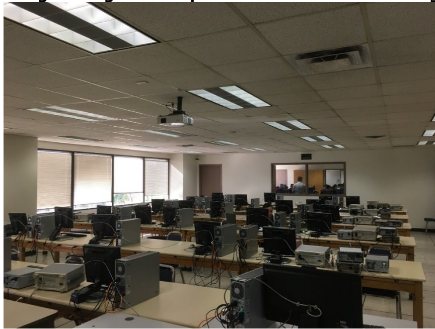
Figure 9: Room Engineering and Computer Science-411 with Old Lighting Fixtures
