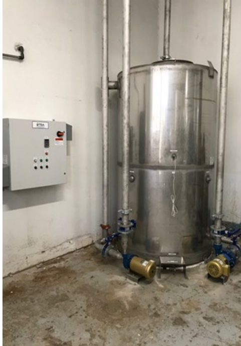
Figure 9: Buffer Tank and Pumps
