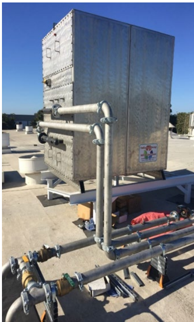
Figure 10: Economizer Roof Mounting
