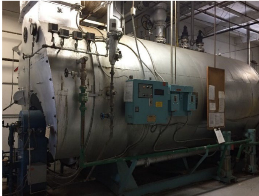
Figure 5: Project Site Dixon Boiler
