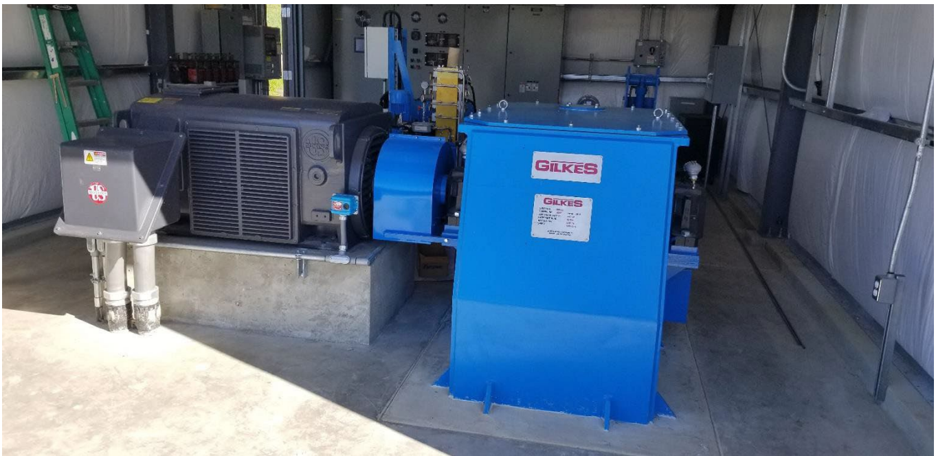
Gilkes Pelton Wheel Turbine, generator and electrical equipment inside new powerhouse building at Ione Reservoir.
