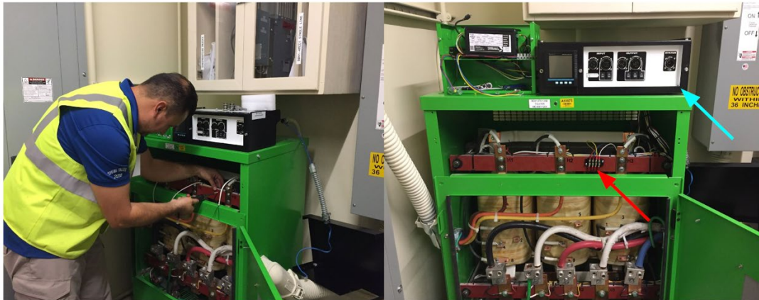
Figure 6a: Transformer Temperature Sensor Installation
