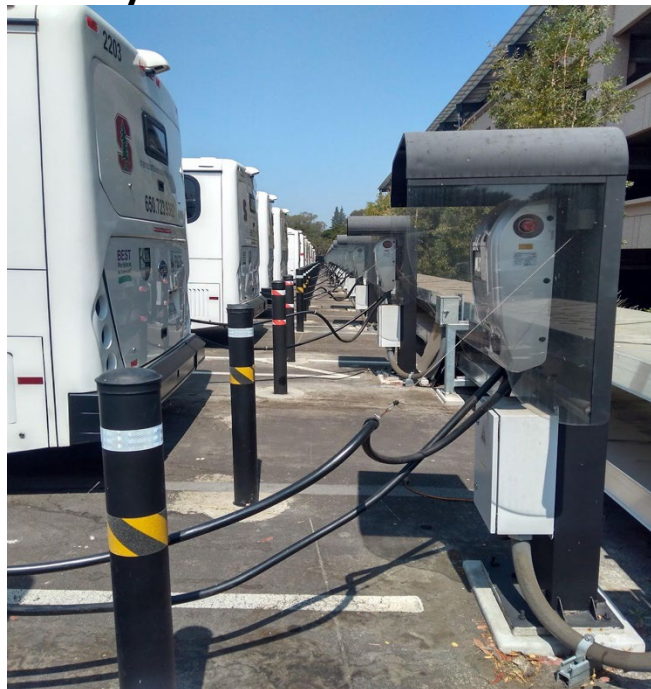
Figure A-1: Stanford bus yard with buses connected to the charging stations
