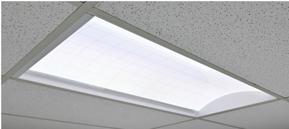
Figure 47: Installed Volumetric LED Troffer in a Switched-on State
