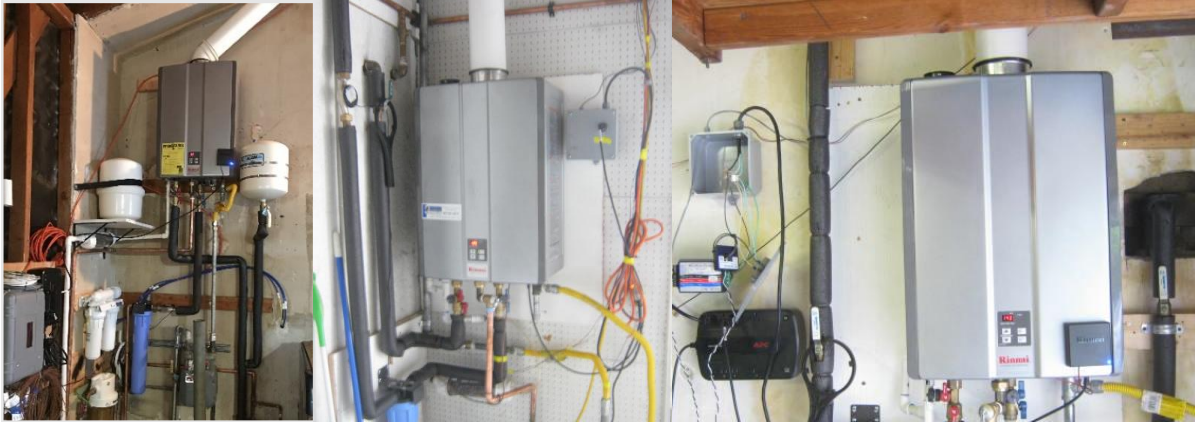
Figure 9: High-Efficiency Tankless Water Heaters Installed as Retrofits at Host Sites #1, #3, and #4
