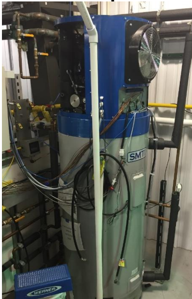
Figure 20: Third Generation Gas Heat Pump Water Heating Testing at GTI in 2016
