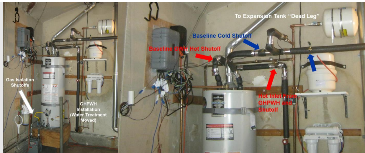
Figure 8: Baseline Monitoring Equipment and Preparations for Gas Heat Pump Water Heater Installation at Site #1
