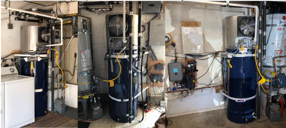
Figure 15: Sites #2, #3, and #5 – Gas Heat Pump Water Heater Installations
