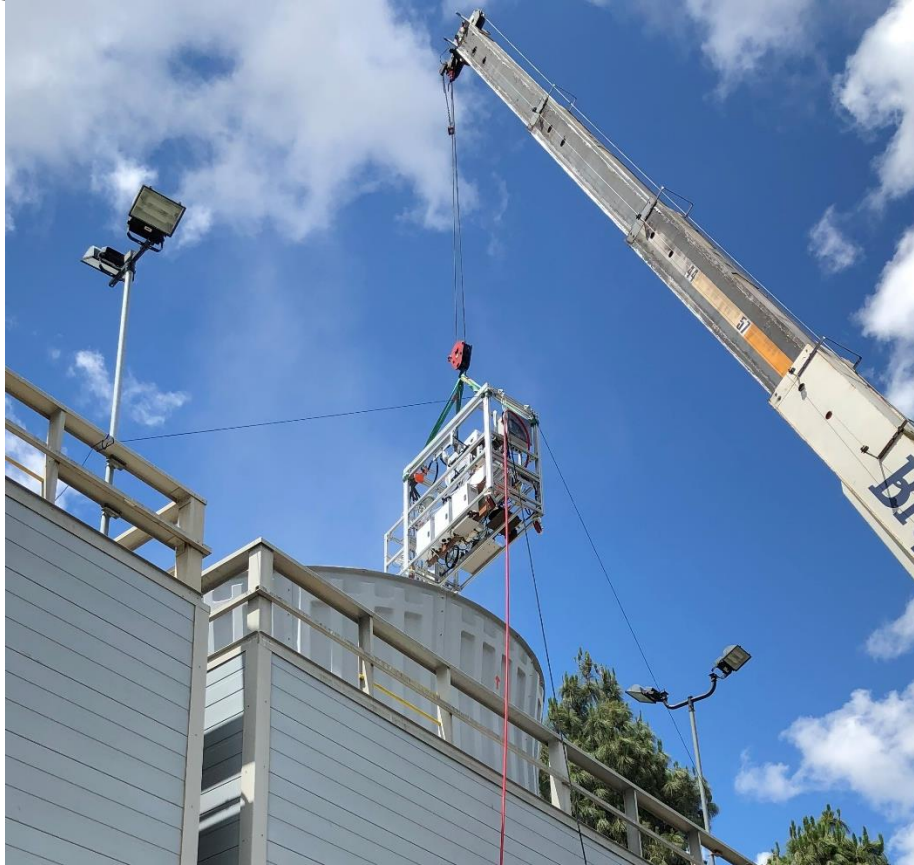
Figure 2: Instrument Package in Place Above a Cooling Tower
