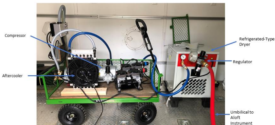
Figure 5: Dry Air Generation Equipment Including Compressor, Aftercooler, Dryer, Regulator, and Umbilical Hose
