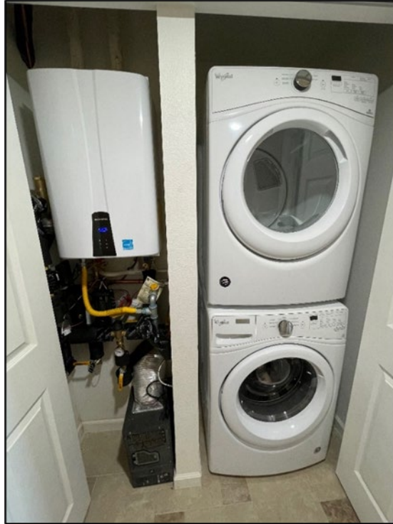
Figure 12: Tankless Water Heater and Washer/Dryer
