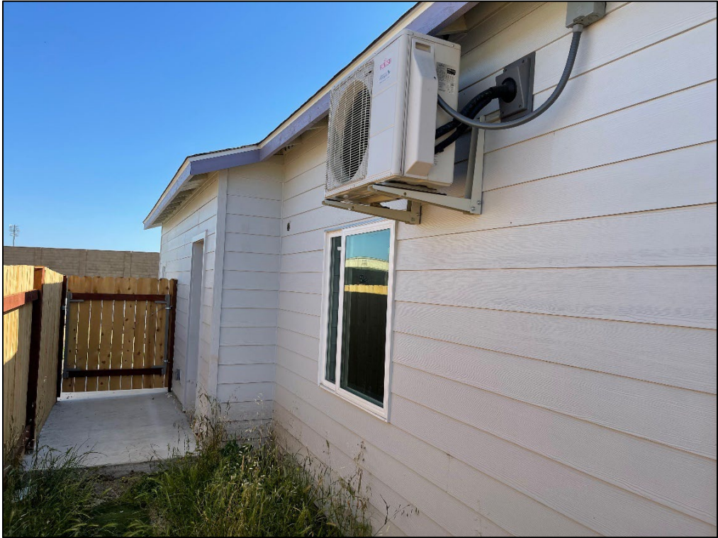
Figure 9: All-Electric Home’s Installed Heat Pump
