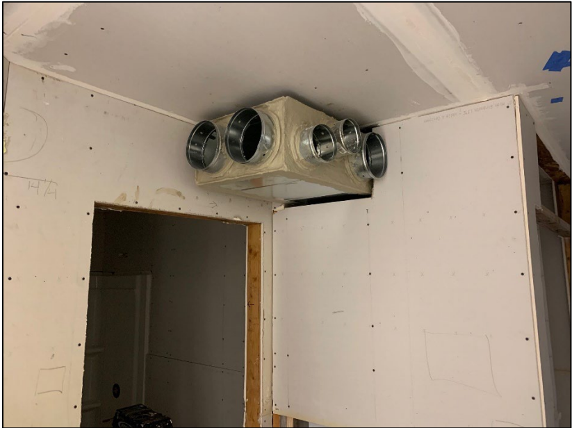
Figure 10: HVAC Duct Distribution Manifold
