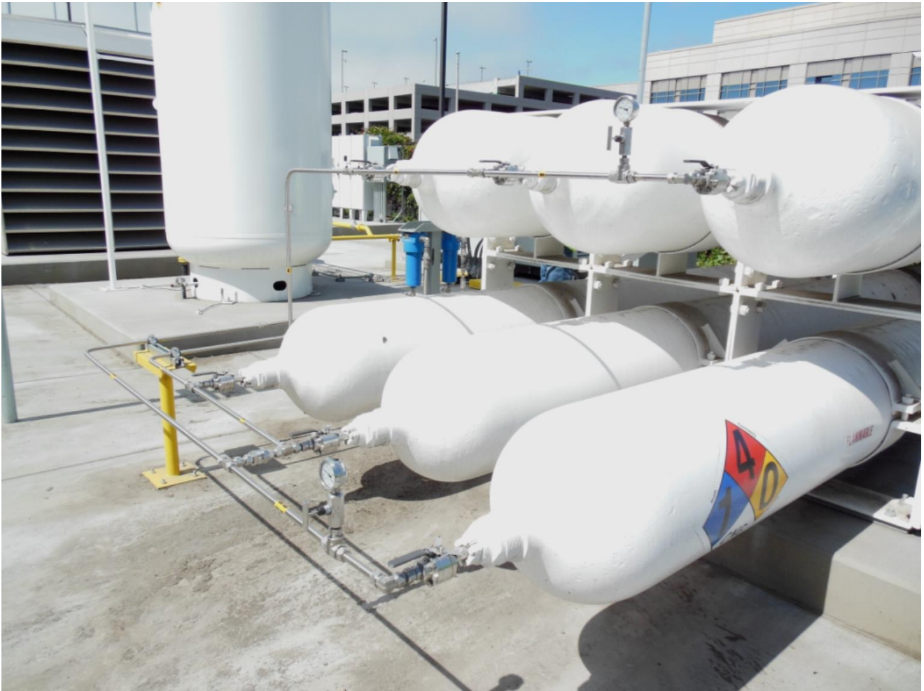
Figure 10: Five Renewable Natural Gas and One Pipeline Natural Gas High Pressure Tanks and Blend Line
