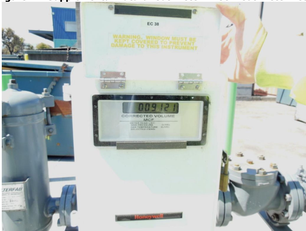
Figure 14: Supplemental Natural Gas Meter –PG&E Gas Meter EC38
