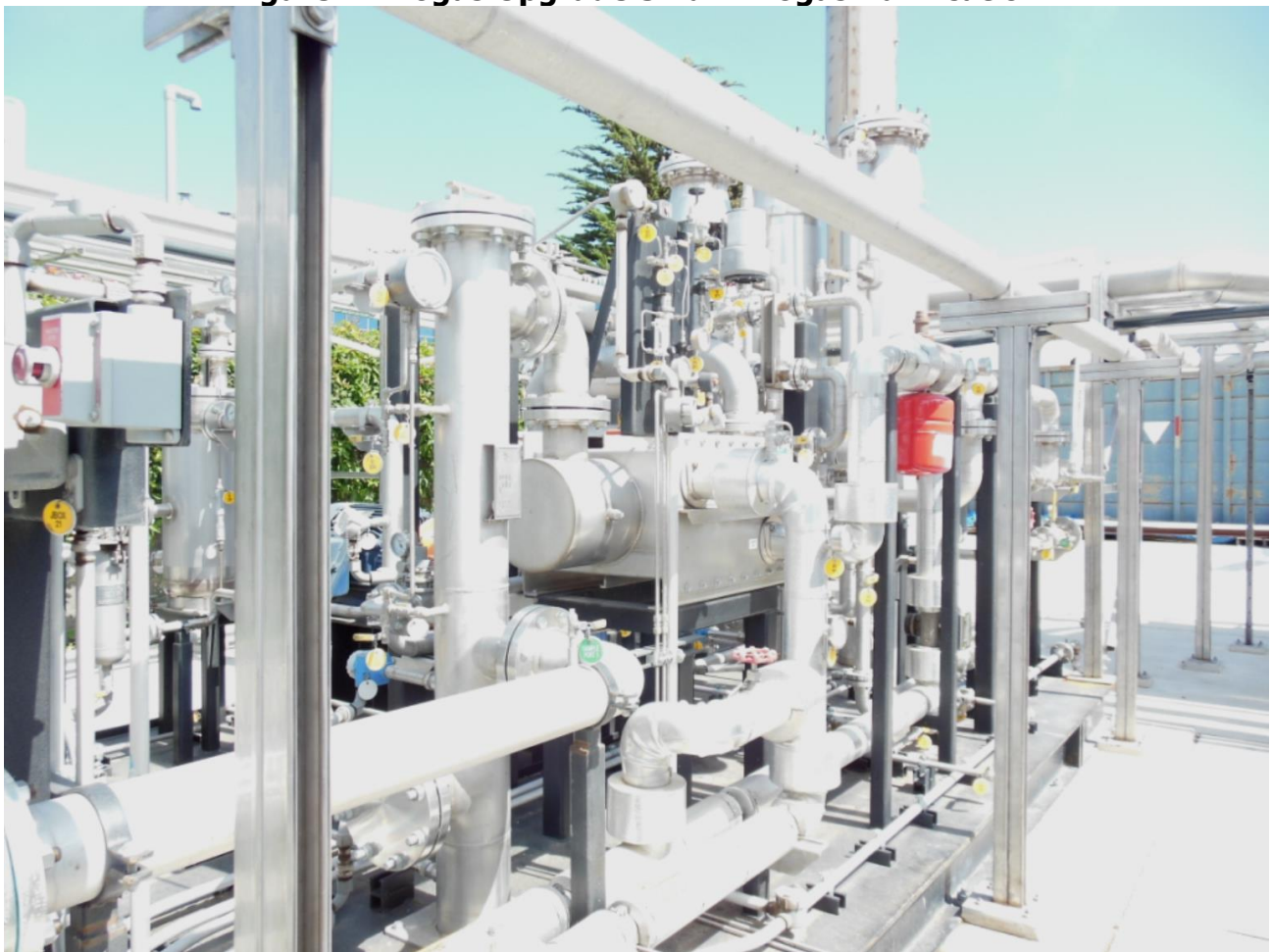
Figure 7: Biogas Upgrade Skid – Biogas Purification
