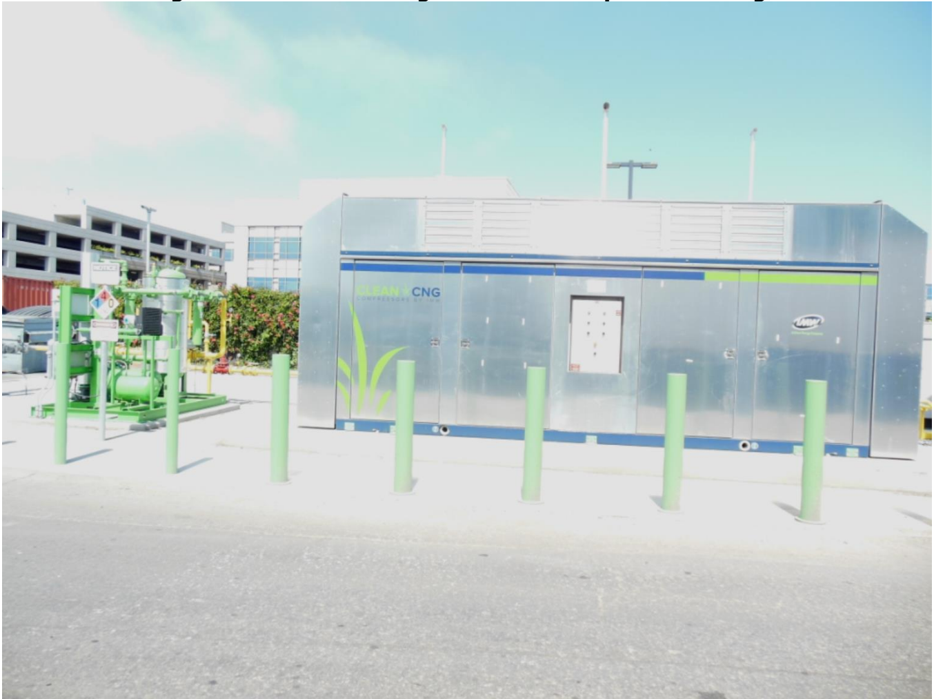
Figure 9: Natural Gas High Pressure Compressor 5-Stage
