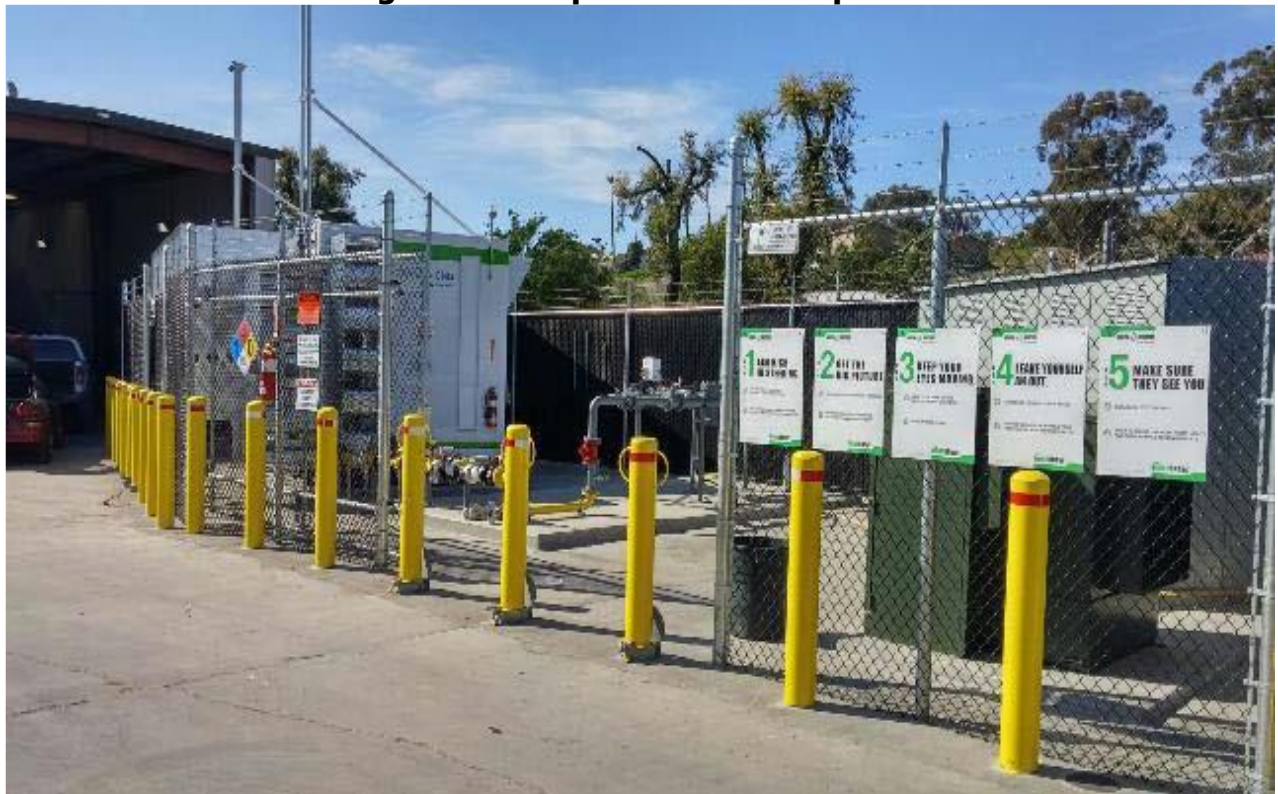
Figure 2. Completed CNG Compound
