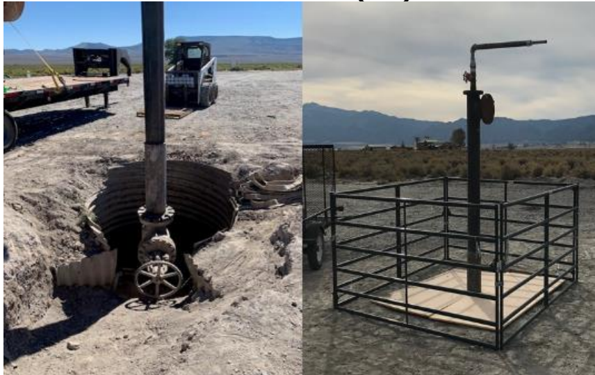
Figure 4: WME-E1 Wellhead Flow Valve (left) and Secured Well (right)
