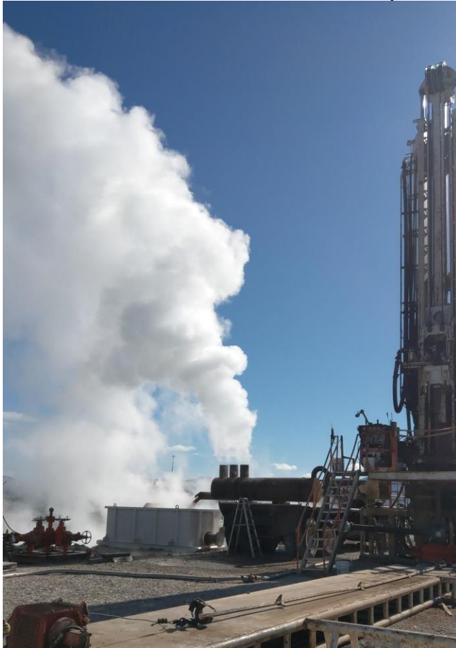
Figure 21: Well WME-E1 Clean-Out Flow, June 2019
