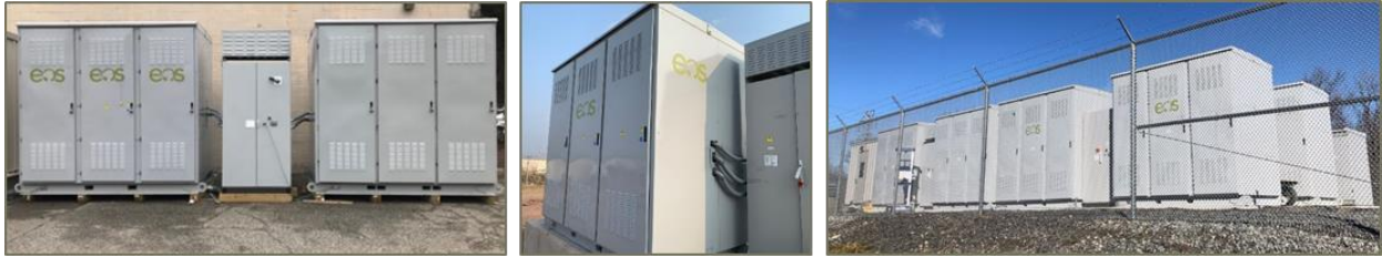
Left to right: (1) testing Eos' first Gen2 system at its HQ in Edison, NJ, (2) 120kWh pilot system deployed in India, (3) 1MWh system at the PSE&G microgrid in New Jersey.
