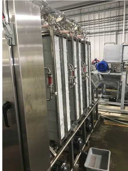
Figure 14: Stacks of PFO-100 Elements Within RC6 System
