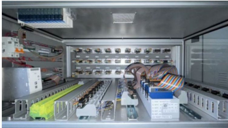
Figure 9: Electrical Panel for Manifold. Image of the Electrical Panel Build under the Manifold
