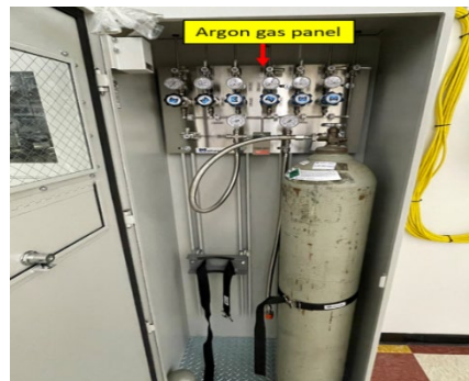
Figure 3: Installed Argon Gas Cabinet Panel. Argon Gas Cabinet Panel with Multiple Delivery Lines for Different Pressure Requirements.
