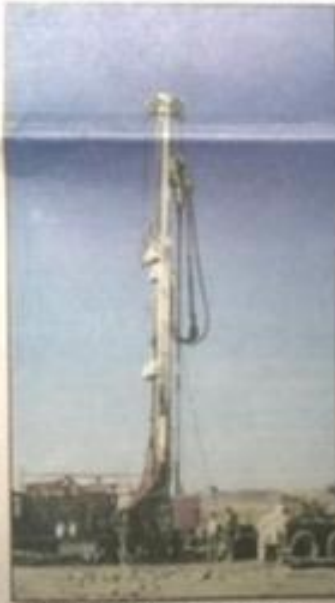
THE well rig that has just drilled to 900 feet in depth for the Western Mountain Energy project.
