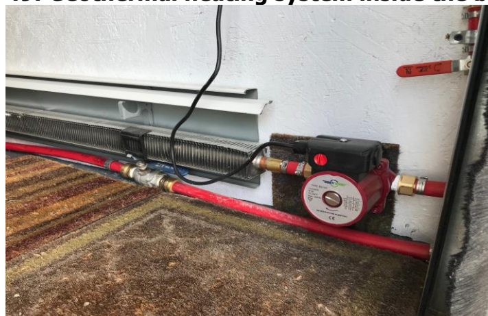
Figure 49: Geothermal heating system inside the building.
