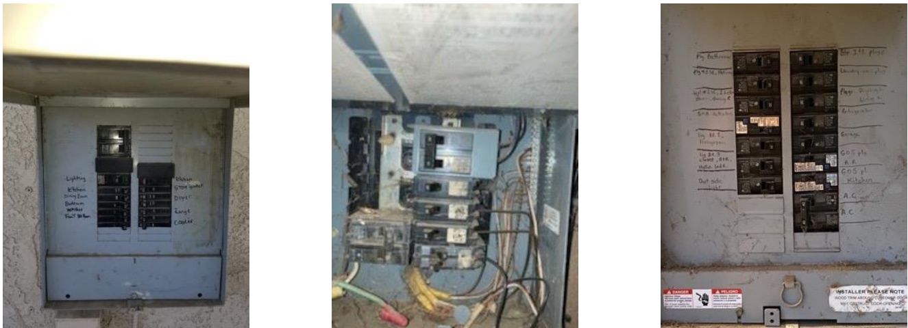
Figure A-13. Photos of Electrical Panels
