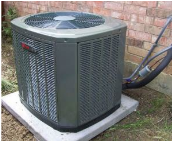
Figure 79. Outdoor Compressor/Condenser Unit of a Split System Mounted on the Ground.
