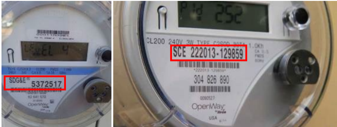
Figure 25. Electric Meters for SDG&E and SCE.
