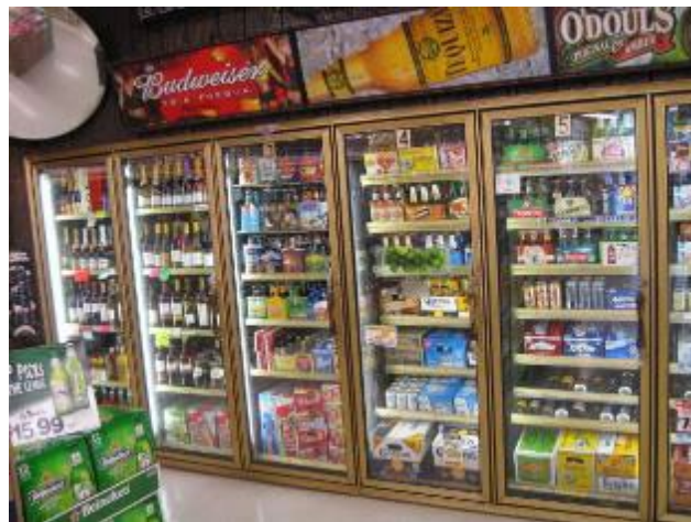
Figure 117. Refrigerated Glass Door Cases served by Central/Remote Compressor Rack (not in picture).
