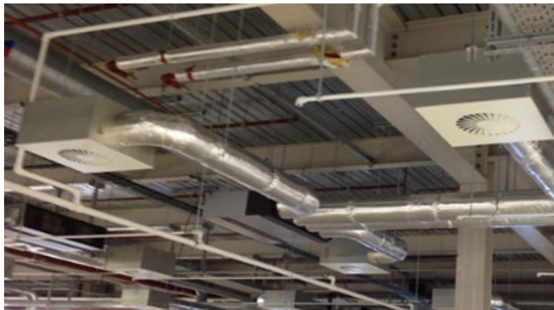
Figure 80. Split System Indoor Fan Coil with Ducting.
