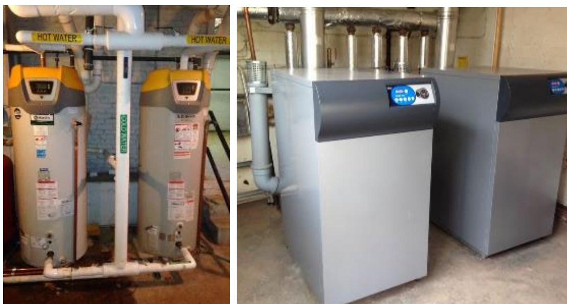
Figure 92. Gas Water Heaters.
