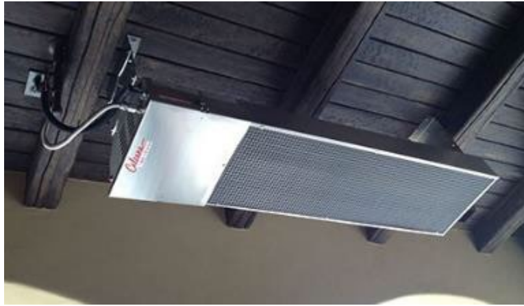
Figure 64. Ceiling Mounted Gas-fired Infrared Heater (not on).
