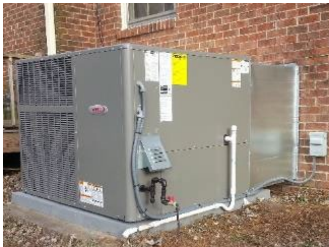
Figure 52. Gas Packaged Unit at ground level (supplying heating and cooling).
