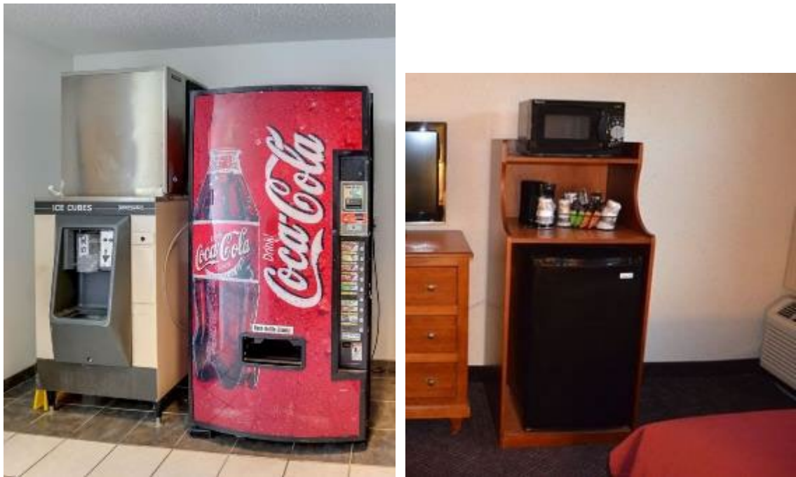
Figure 122. Self-Contained Ice Maker and Drink Vending Machine (left), Room Refrigerator (right).
