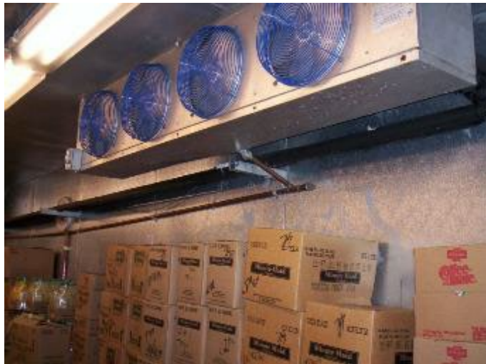
Figure 120. Evaporator Fan Unit in Walk-In Cooler served by Central/Remote Compressor Rack, not shown.
