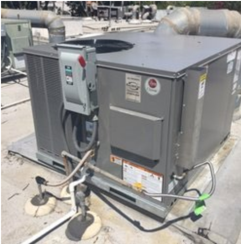
Figure 50. Rooftop Gas Packaged Unit (supplying heating and cooling).
