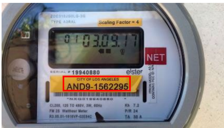
Figure 27. Electric Meter for LADWP.
