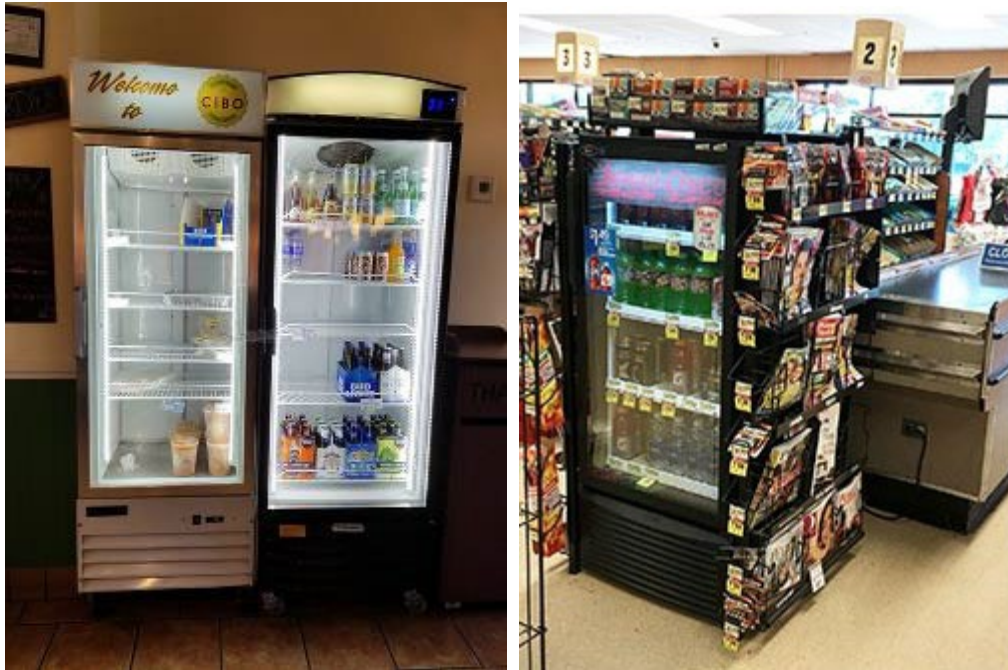
Figure 121. Self-Contained Refrigeration Display Cases.
