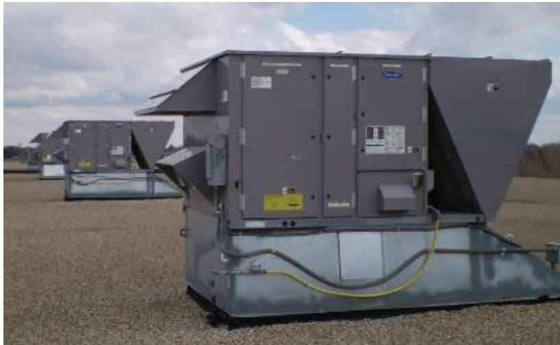
Figure 51. Rooftop Gas Packaged Unit (supplying heating and cooling).
