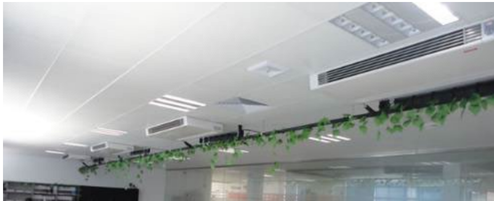
Figure 82. Split System Indoor Fan Coils Surface Mounted without Ducting.
