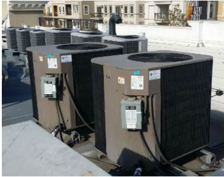
Figure 78. Outdoor Compressor/Condenser Unit of Multiple Split Systems Mounted on a Roof.
