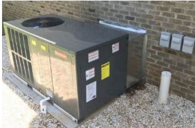
Figure 55. Packaged Heat Pump Unit at ground level (supplying heating and cooling).
