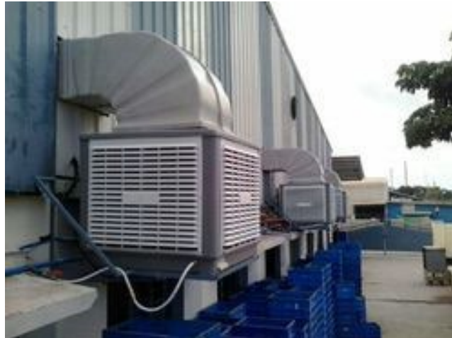
Figure 89. Side Mounted Evaporative Coolers.
