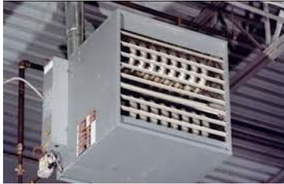
Figure 61. Gas-fired Heater mounted in High Bay Ceiling area.
