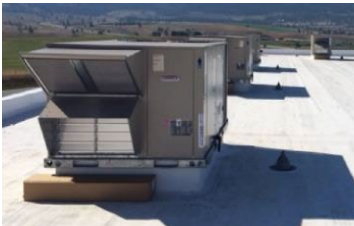
Figure 74. Rooftop Packaged Air Conditioning Units.
