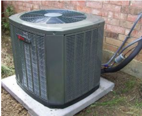
Figure 57. Outdoor Compressor/Condenser Unit of a Split System Heat Pump Mounted on the Ground.
