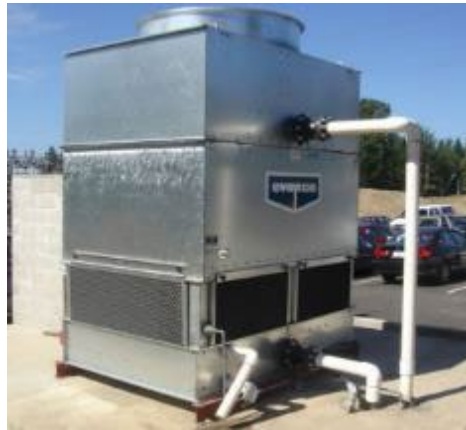
Figure 72. Water Cooling Tower, Small.
