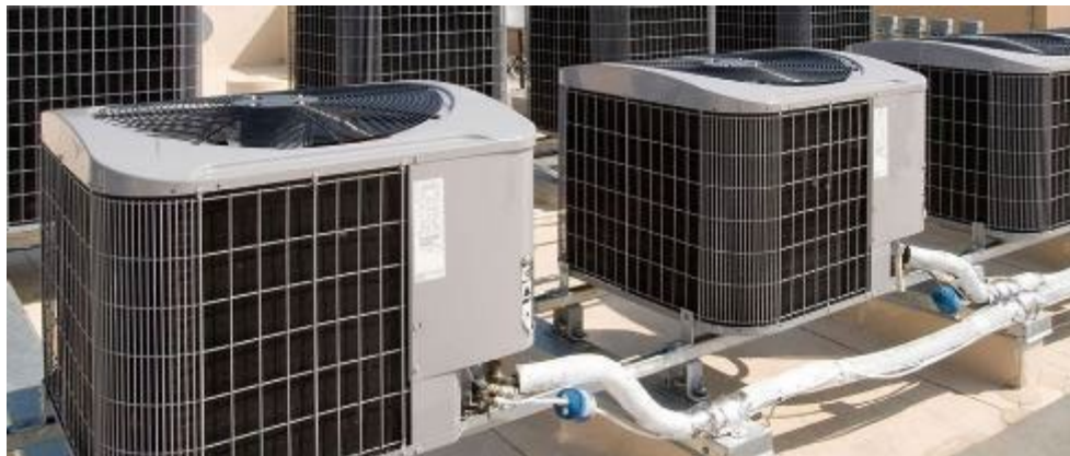
Figure 56. Outdoor Compressor/Condenser Unit of a Split System Heat Pump Mounted on a Roof.
