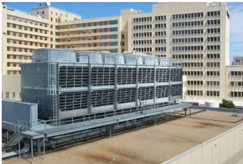
Figure 73. Water Cooling Tower, Large.
