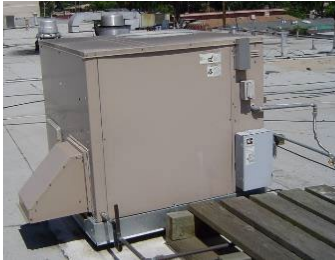
Figure 76. Small Rooftop Packaged Air Conditioning Unit.
