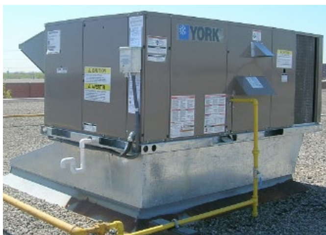
Figure 75. Rooftop Packaged Air Conditioning Unit (with gas heat).
