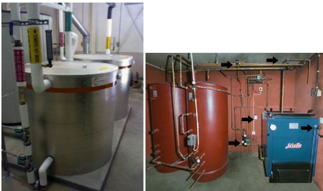
Figure 95. Solar Hot Water Storage Tanks.
