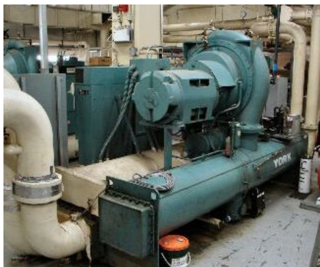
Figure 67. Centrifugal Chillers in Mechanical Room.
