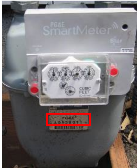
Figure 28. Natural Gas Meter (PG&E) with a SmartMeter attachment.
