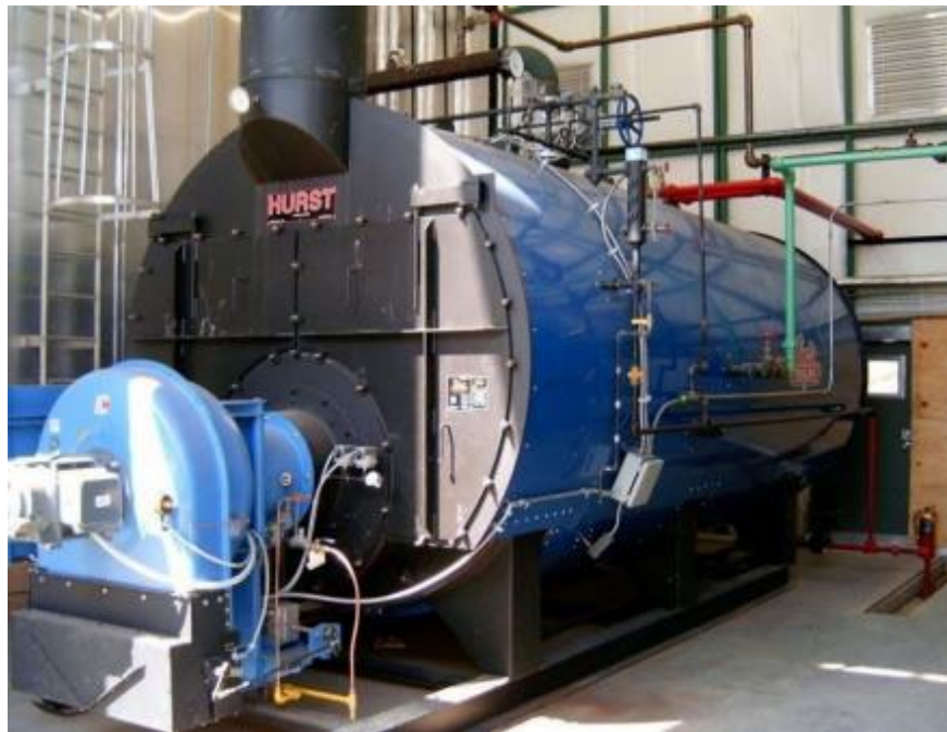
Figure 48. Large Gas Boiler for Heating Water to Heat Space.
