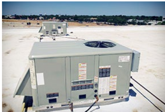
Figure 53. Rooftop Heat Pump Packaged Unit (supplying heating and cooling).
