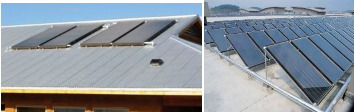
Figure 94. Solar Water Heater Panels.
