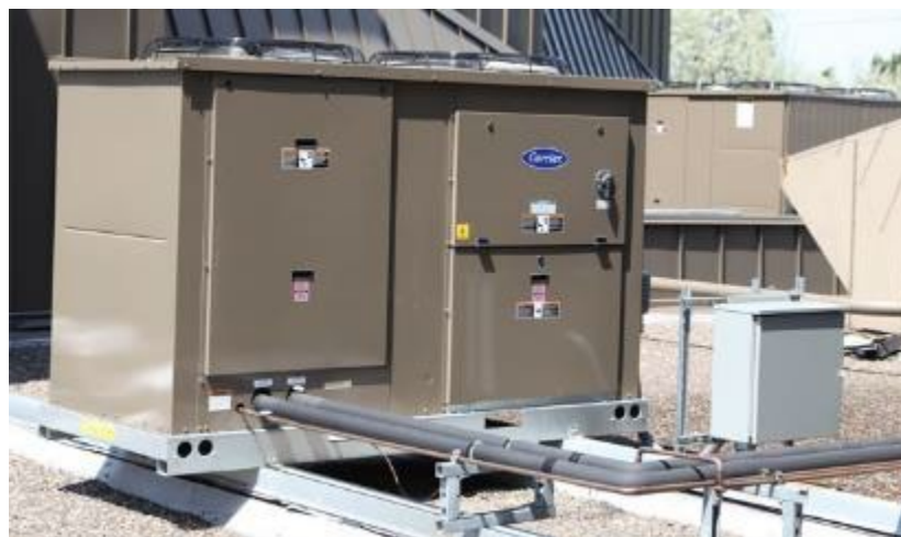
Figure 77. Outdoor Compressor/Condenser Unit of a Split System Mounted on a Roof.
