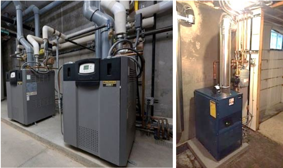
Figure 49. Medium (left) and Small (right) sized Boilers for Heating Water to Heat Space.
