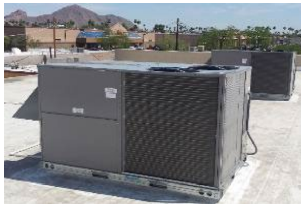
Figure 54. Rooftop Heat Pump Packaged Unit (supplying heating and cooling).
