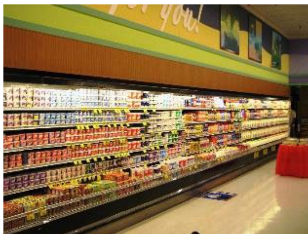
Figure 118. Refrigerated Open Cases served by Central/Remote Compressor Rack (not in picture).
