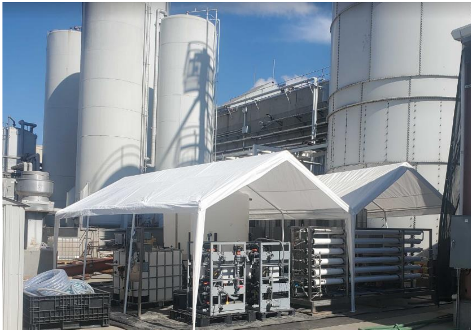
Figure 10: PFO Recycler System at Frito-Lay, Modesto
