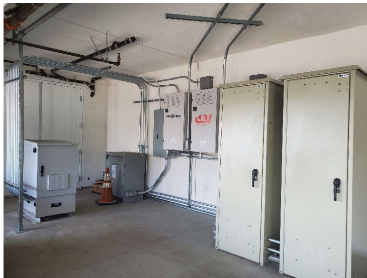
Figure 6: Installed CE+T Stabiliti 30C3 Inverter Units (Left) and Enclosed EnergPort L3060 Batteries (Right)
