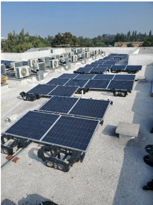
Figure 4: Bifacial Solar Installation at Project Site
