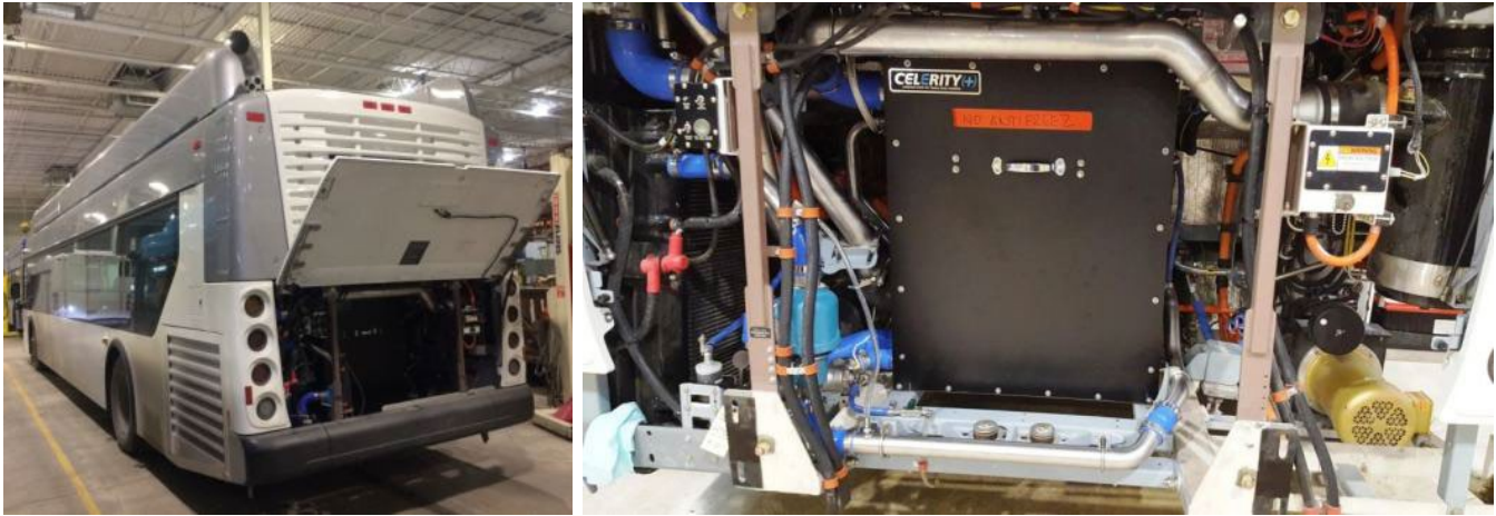
Figure 11: Hydrogenics Celerity Plus Subassembly Installed in Bus Engine Bay
