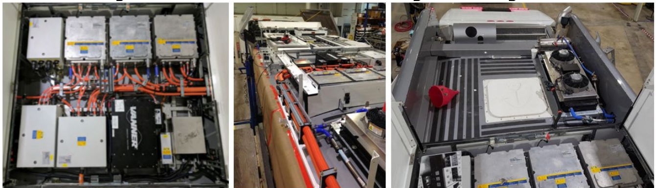
Figure 30: Details of the electrical wiring and cooling lines
