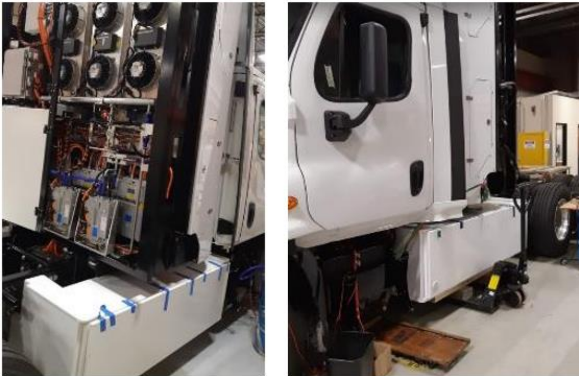
Figure 16: ACTIA High Volt Battery Modules Installed on Truck
