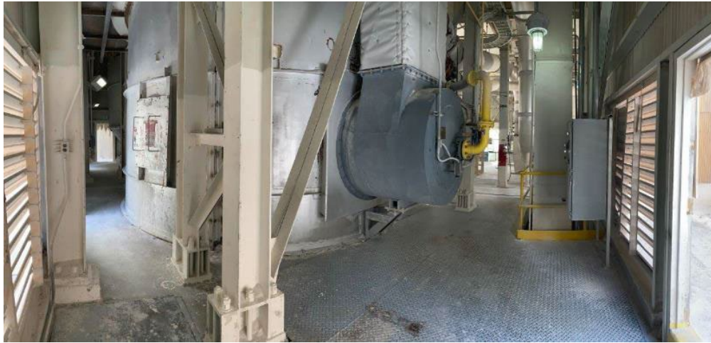
Figure 9: Bottom of the gypsum kettle at USG showing the burner
