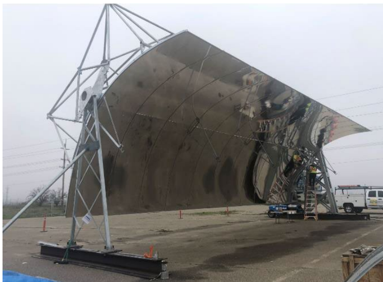
Figure 24: Parabolic trough with absorber support structures installed at UCM
