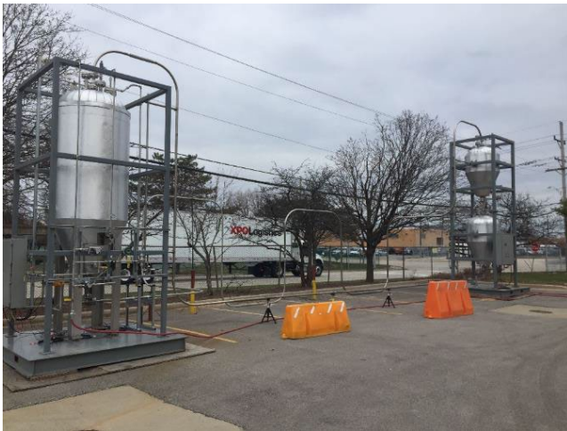
Figure 50: Piping layout between the storage hopper skid (left) and stacked receiving and lock hopper skid (right)
