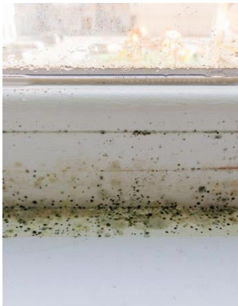
Figure 9: Mold on Windowsills can Lead to Negative Health Impacts
