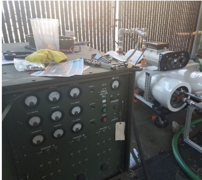
Figure 20: Military Grade Electrical Load Bank
