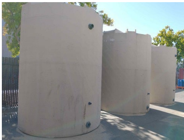
Figure 21: 4,500-Gallon Storage Tanks for the Draw Solutions and Working Fluid
