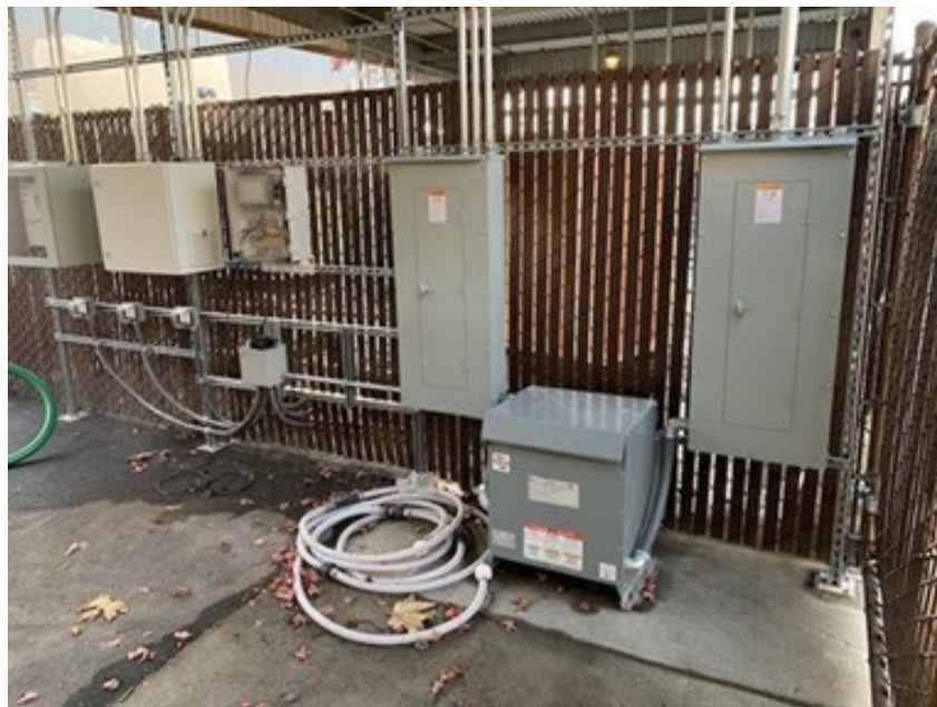
Figure 19: Electric Supply and Dedicated Control System
