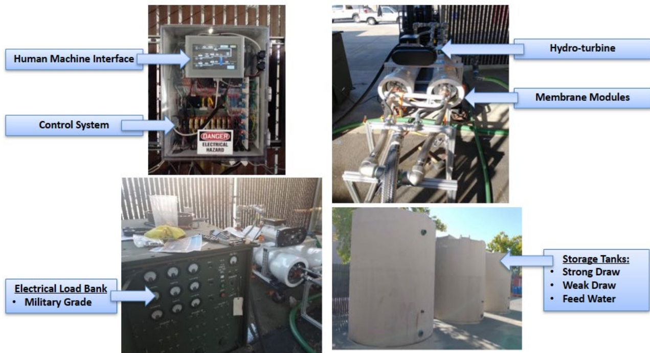
Figure 25: HMI, Load Bank, Membrane Modules and Storage Tanks
