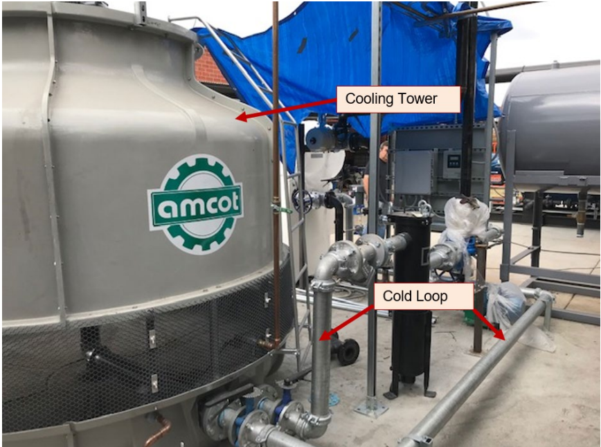
Figure 8: Piping to and from the cooling tower to the ORC system (cold loop)
