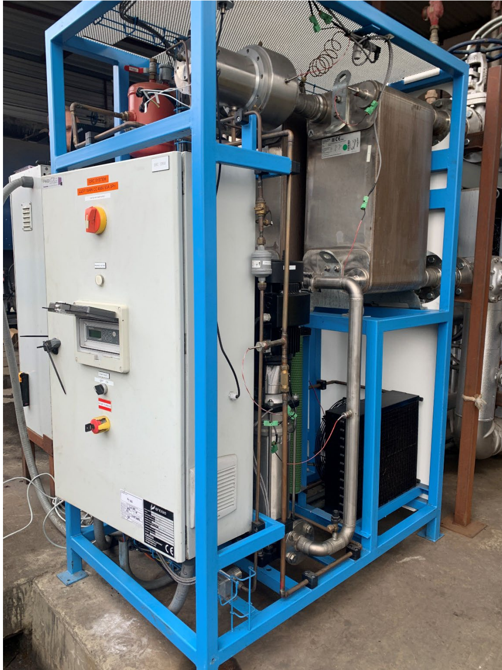
Figure 14: ORC system during commissioning
