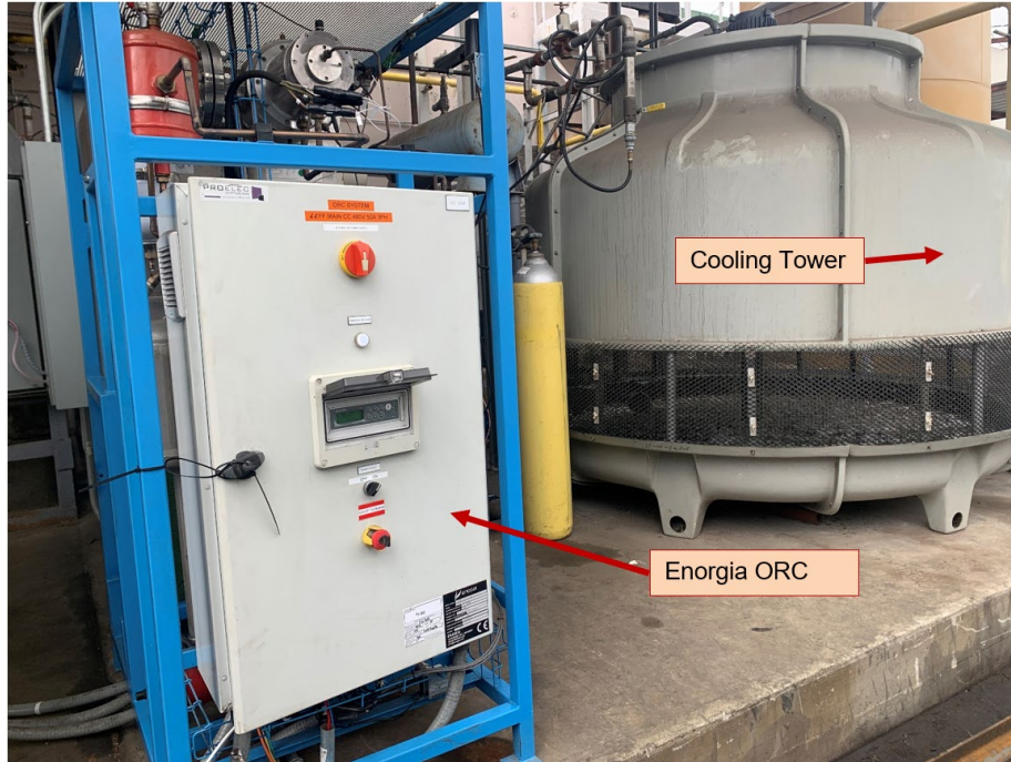
Figure 5: Installed 20 kW Enogia ORC system and Amcot cooling tower
