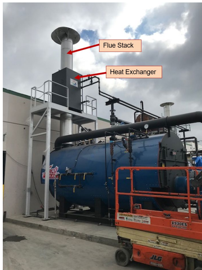
Figure 6: Hurst steam boiler and flue gas heat exchanger
