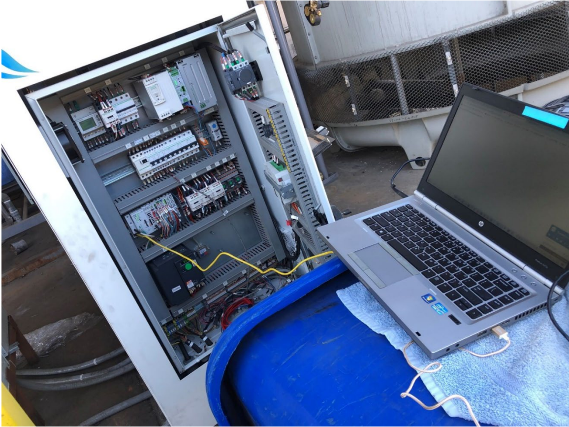
Figure 12: ORC pre-commissioning system test
