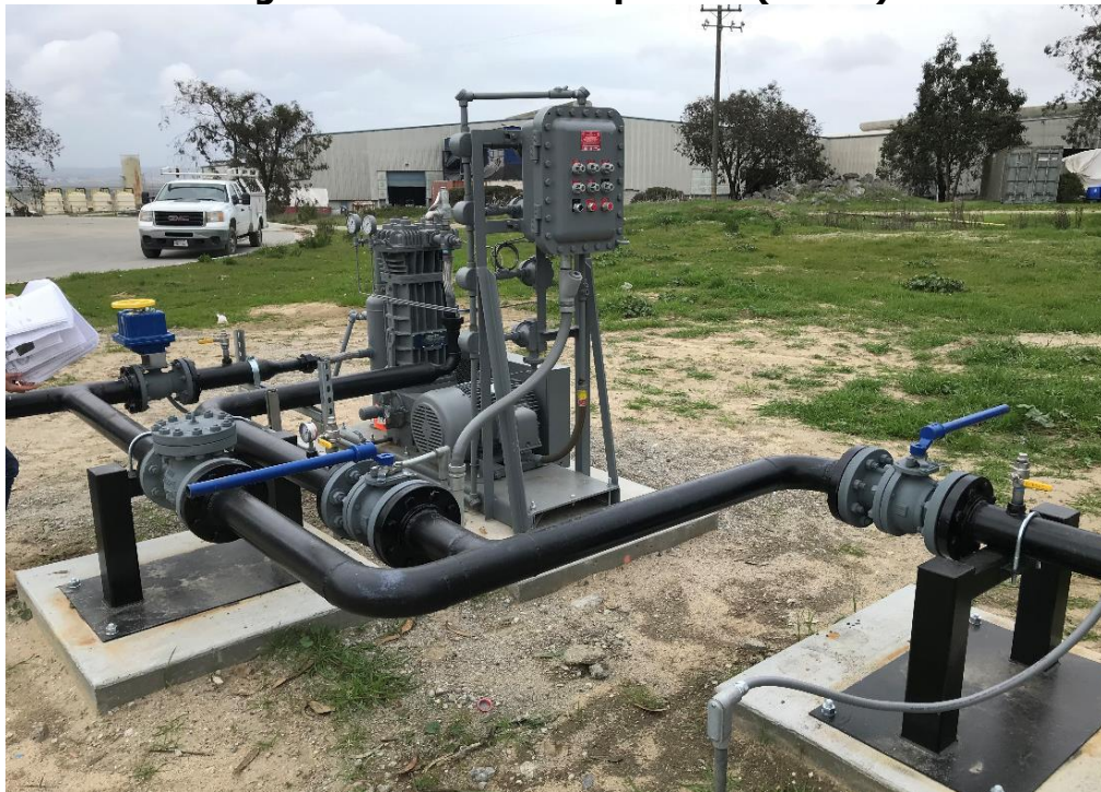
Figure 3: Booster Compressor (25 HP)
