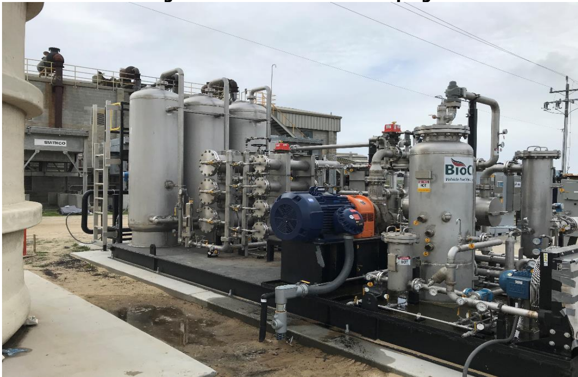
Figure 1: BioCNG™ Skid and Piping
