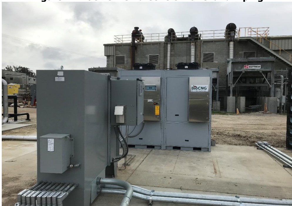
Figure 2: BioCNG™ Skid Control Panel and Piping
