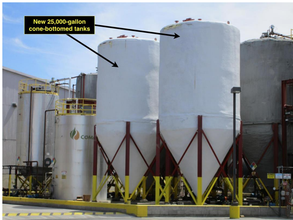
Figure 2: New Storage Tanks for Alternative Feedstocks
