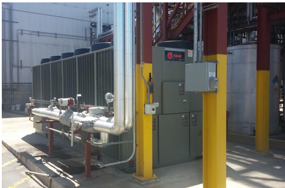
Figure 5: New Chiller for Methanol Recovery and Recycling System
