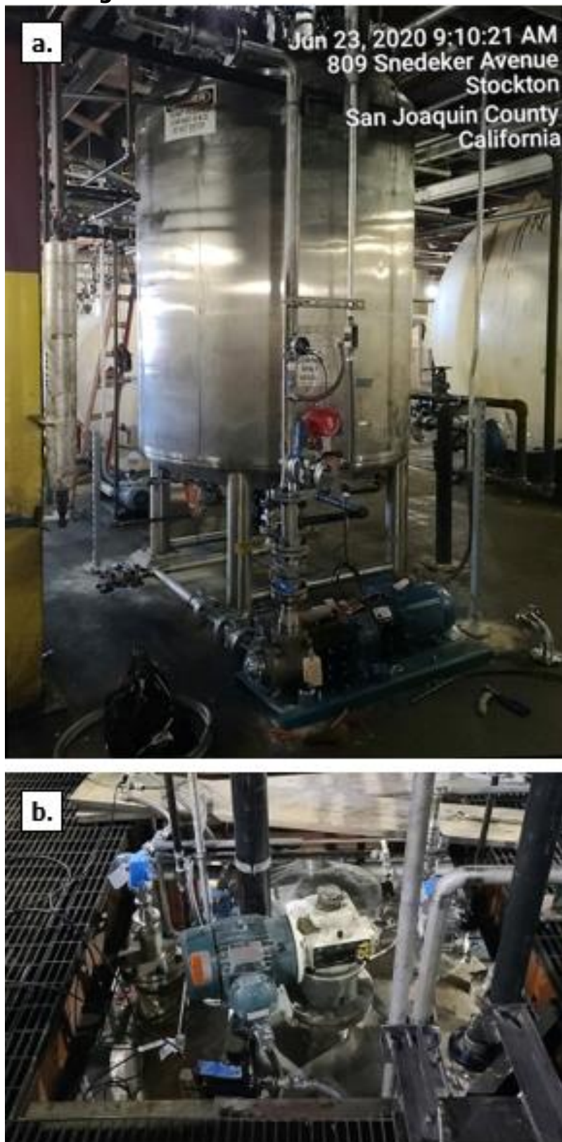
Two views of the new stainless steel reactor: a) the reactor vessel and base from the process room floor; b) the top of the reactor, with mixer motor and instrumentation installed, from the elevated platform in the process room.
