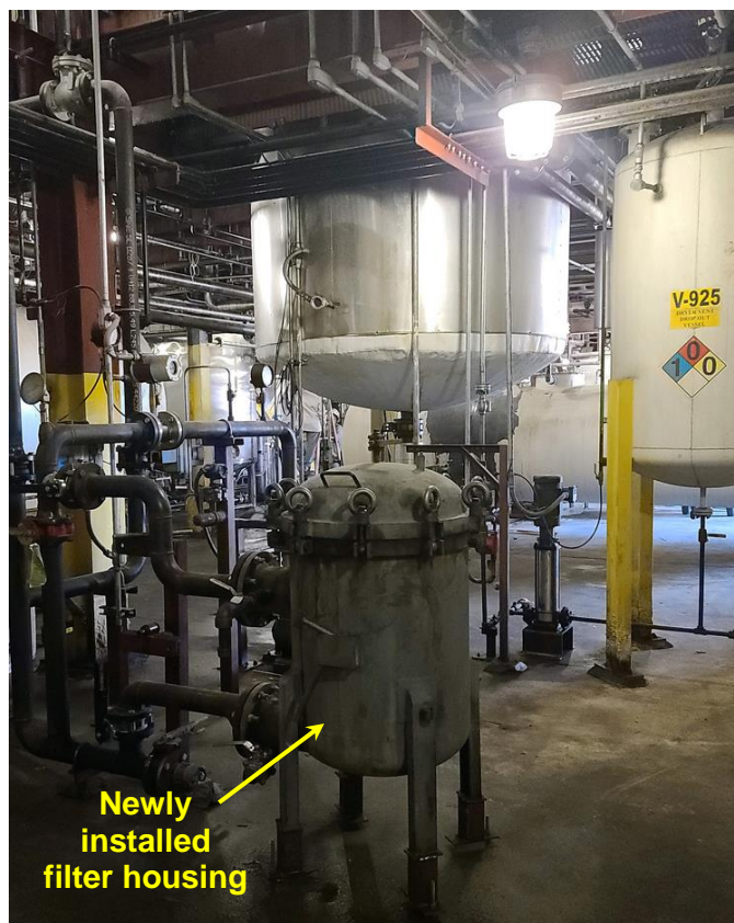
Figure 12: Filter Housing on the Outlet Line from the FAME Dryer
