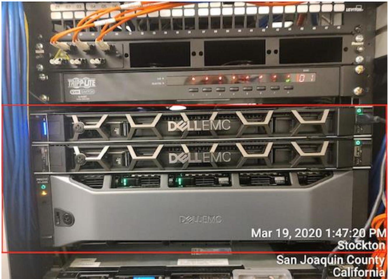
Figure 7: New HMI Servers and Drive Array
