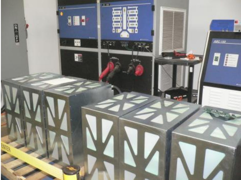
Figure 9: KAM Modules Under Test in TransPower's ESS Lab
