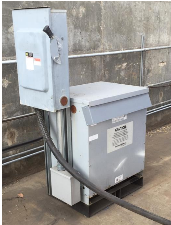
Figure 20: Complete EVSE with Transformer and Charge Control Box
