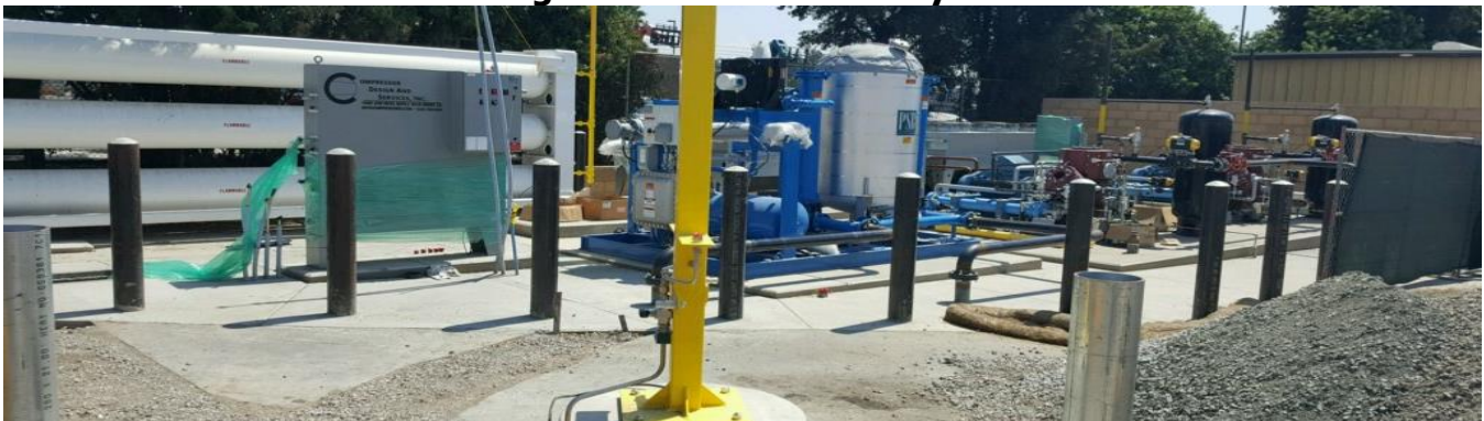
Figure 2: Natural Gas Dryer
