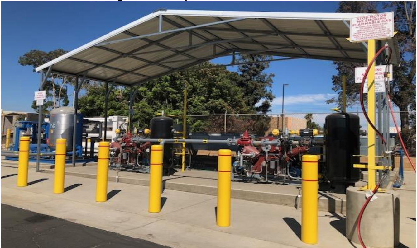
Figure 10: Complete CNG Infrastructure
