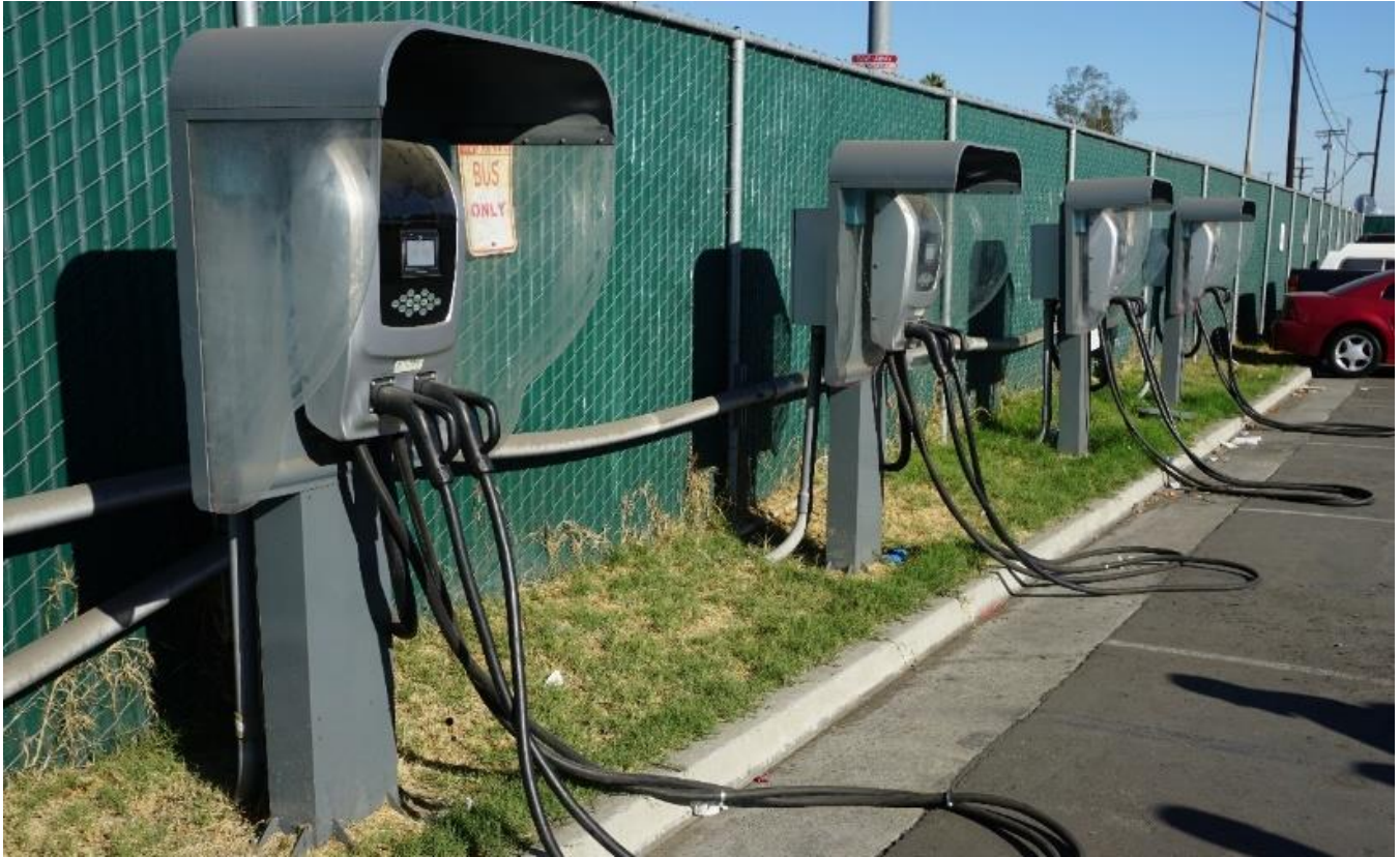
Figure 8: LADOT Depot Chargers
