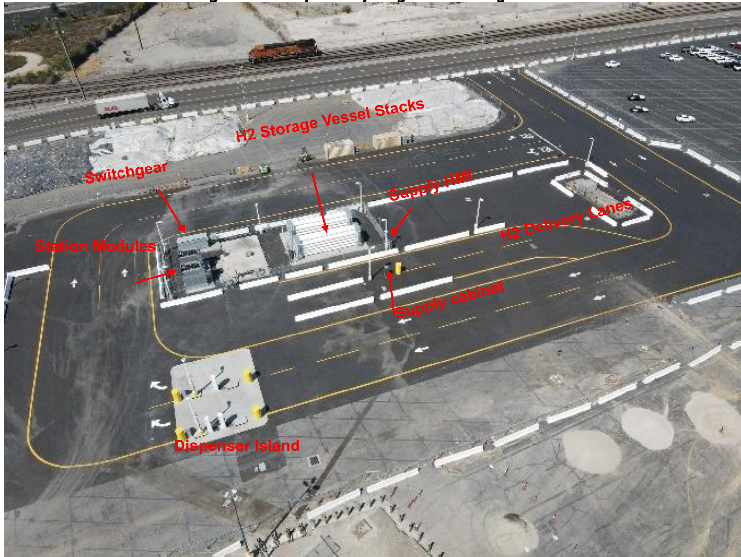
Figure 6. Complete Hydrogen Refueling Station
