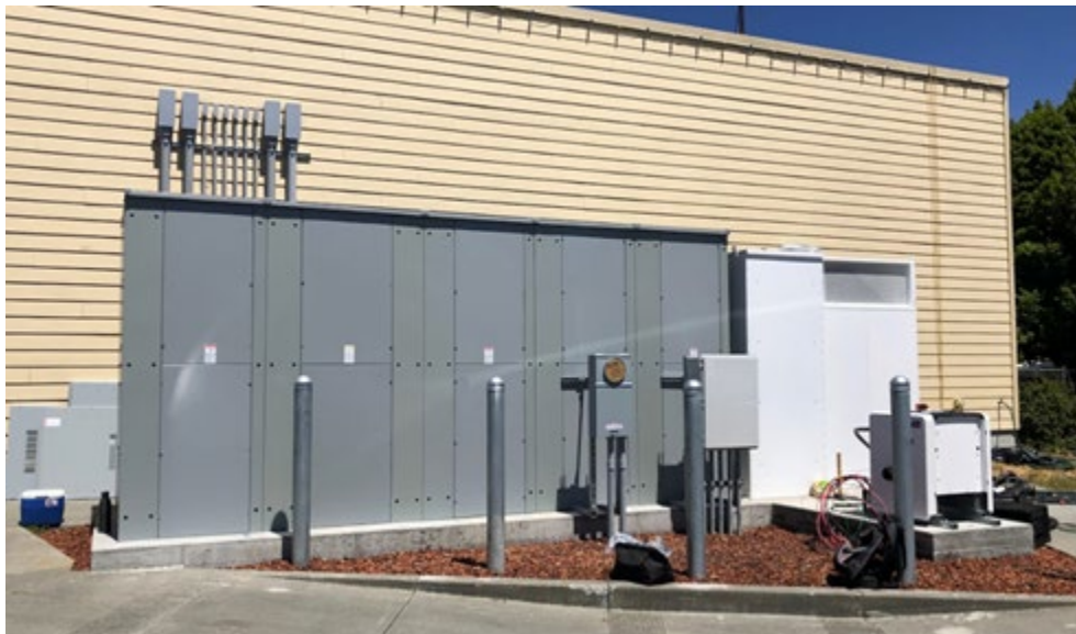
Complete equipment lineup, shown on equipment slabs
