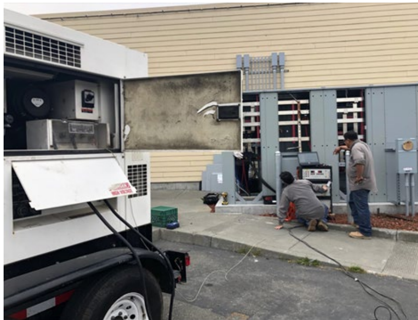
The team testing the monitored, controlled, motorized breaker.
