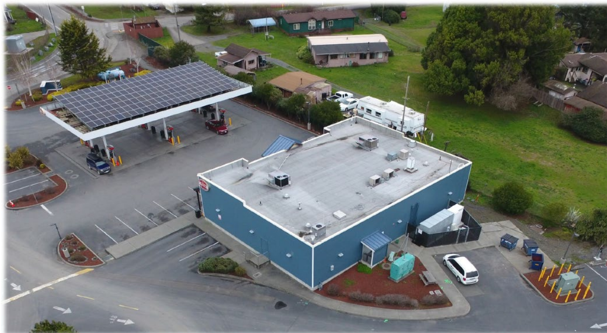
Microgrid hardware includes PV array on canopy and battery storage and switchgear at rear corner of store.
