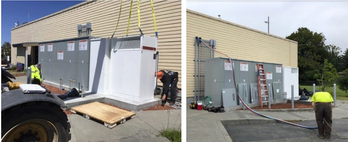
Staff placing the BESS inverter and pulling conductors from inside the C-store to the islanding switchgear.
