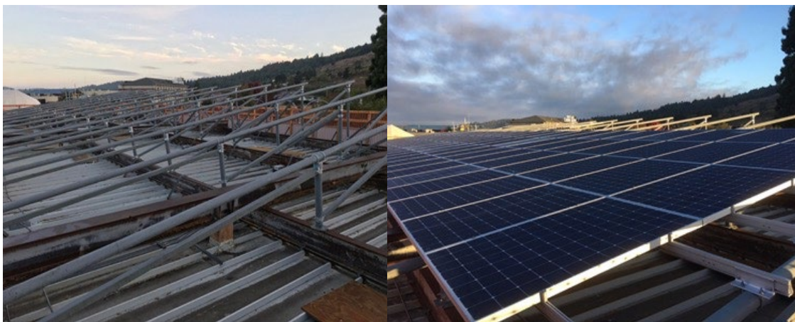
Image on the left shows PV array racking substructure and on the right installed PV modules on the racking structure.
