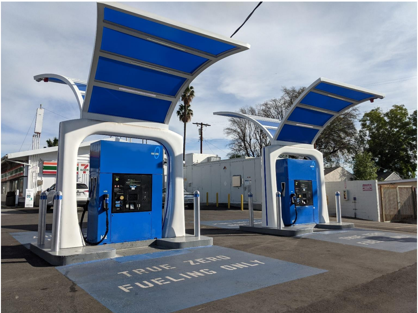
Figure 12: Completed Mission Hills Hydrogen Station
