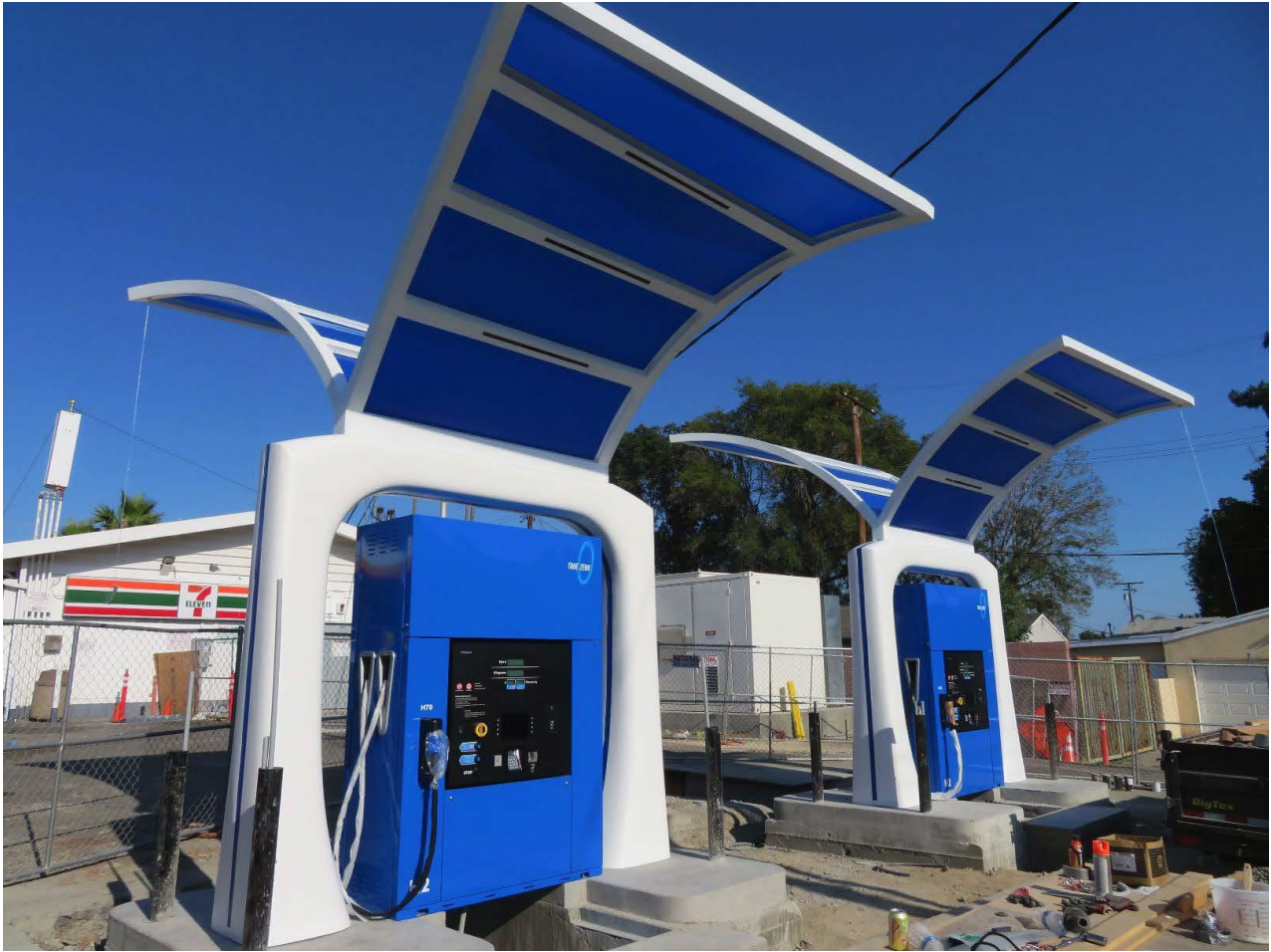
Figure 8: Tatsuno Dispensers Progress at the Mission Hills Station
