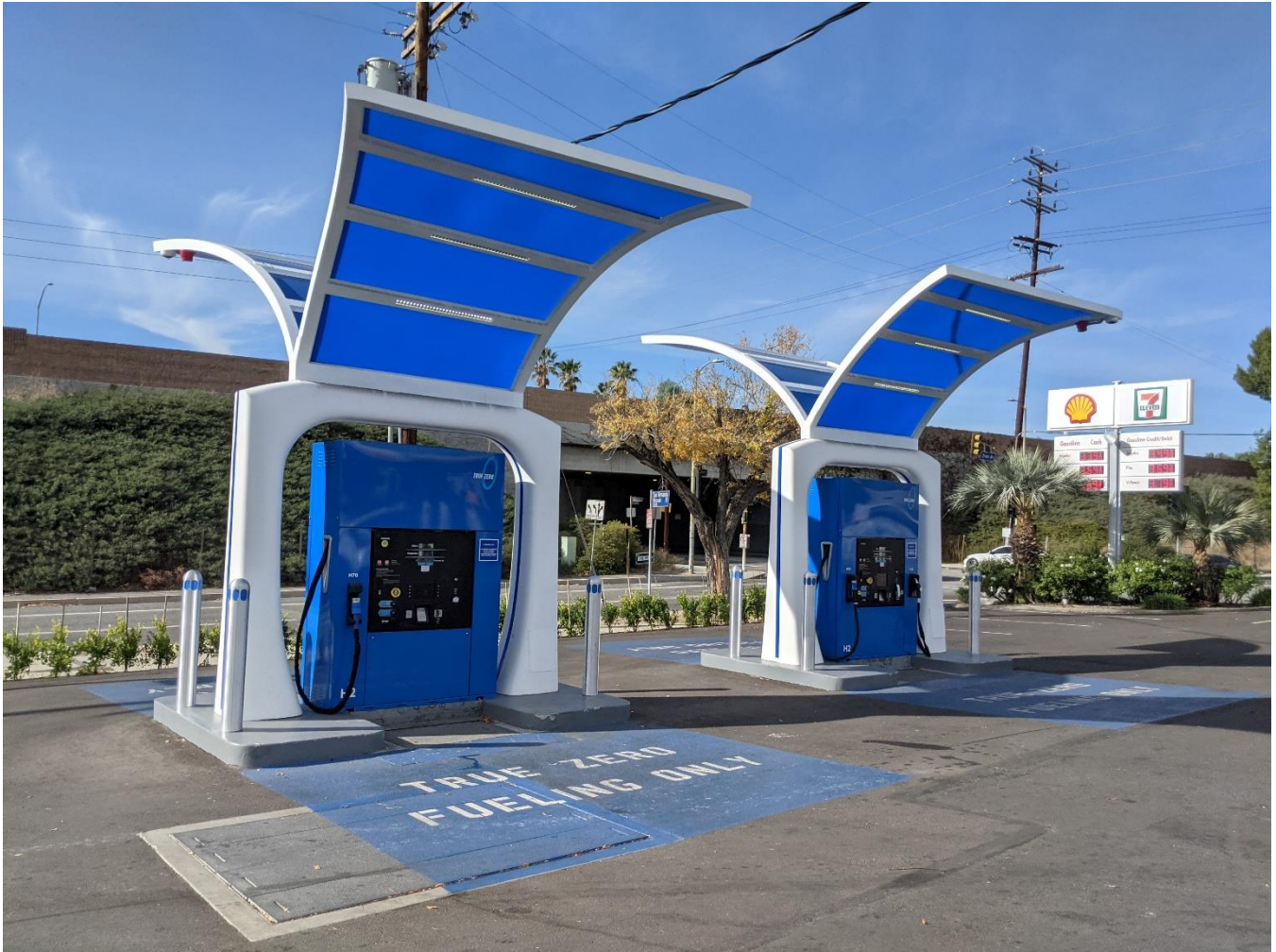
Figure 3: Installed Tatsuno Dispensers With Four Fueling Positions
