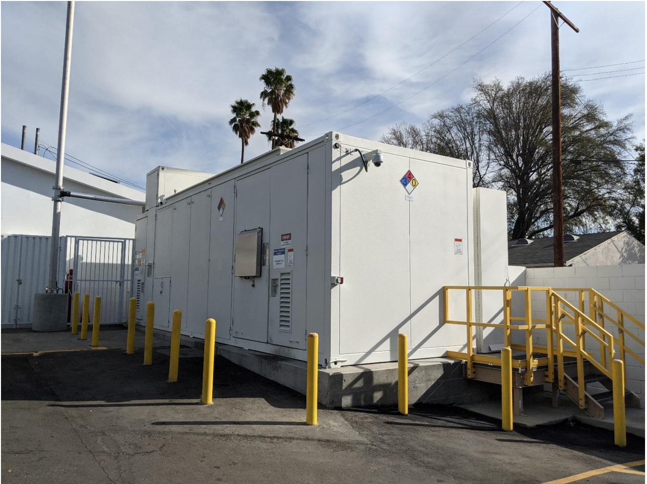
Figure 4: Linde Unit (Compressing and Dispensing Equipment)
